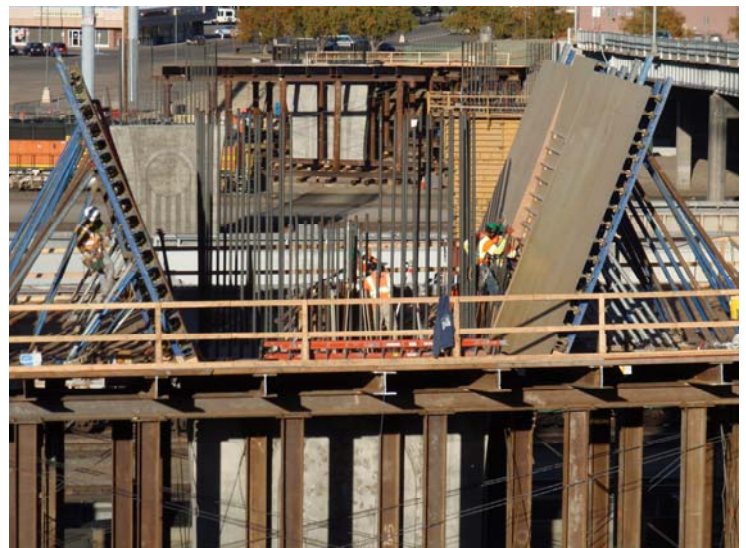
Figure 5 – Pier 3 WB Pier Table Construction – October 28, 2008: The carpenters form the flared portion of the column, which projects out from the typical web slope.
