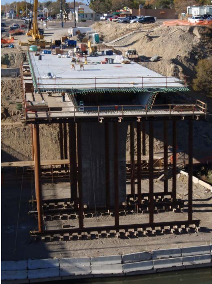
Figure 6 – Span 1 WB CIP Superstructure Construction – October 31, 2008: Flatiron begins to remove the equipment and materials from the deck following stressing and grouting operations. The falsework removal will consist of suspending the stringers from winches, removing the falsework bents, and lowering the stringers to the ground.
