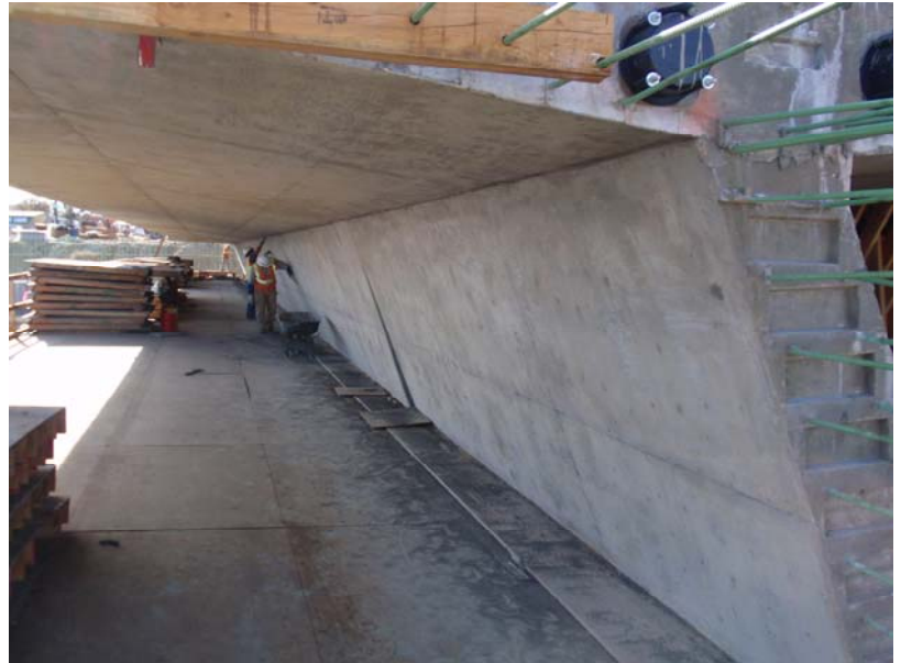
Figure 8 – Span 1 WB CIP Superstructure – November 3, 2008: Workers strip the web and wing forms and prepare the surface prior to lowering the falsework. The shadow visible on the web (between the worker and the cantilever tip) is the extension of the pier as it flares up and transitions into the web.
