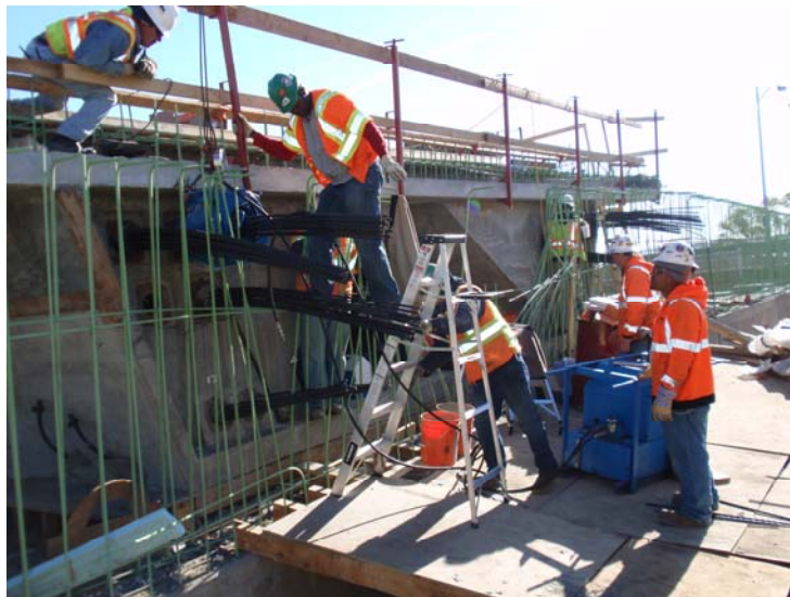
Figure 4 – Span 1 WB CIP Superstructure Construction – October 27, 2008: After stressing all of the transverse tendons and the vertical PT bars in the pier and abutment diaphragms, the PT crew begins stressing the longitudinal tendons in Span 1 WB. In this figure, the crew installs the jack on the 19-strand draped tendons.
