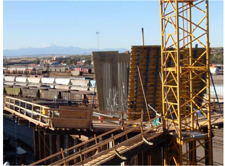
Figure 3 – Pier 3 WB Pier Table Construction – October 23, 2008: The falsework assembly is complete at Pier Table 3 WB and the web forms are partially installed.
