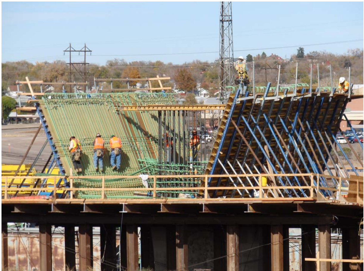
Figure 9 – Pier 3 WB Pier Table Construction – September 30, 2008: The ironworkers begin installing the epoxy coated bottom slab, web, and diaphragm reinforcing.
