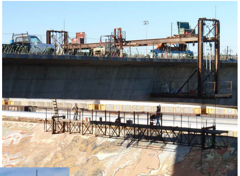
Figure 8 – Bridge Finishing Work – November 4, 2009: Crews work on repairs and pouring back form traveler tie-down holes from the finishing platform in Span 2 WB.
