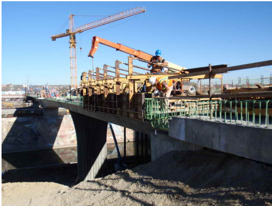
Figure 11 – Span 1 WB Pedestrian Curb Construction – November 18, 2009: Workers set up a 40' section of the pedestrian curb forms at Span 1 WB. Once Flatiron is comfortable with their formwork system, they plan to form and pour the curb in 120' sections.
