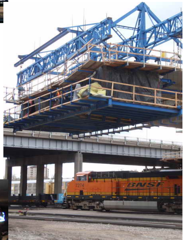
Figure 4 – Cantilever 4 WB Segmental Construction – October 27, 2009: After casting Segment W4-7E, the web forms had to be cut prior to launching the traveler. (The web forms can be seen projecting well below the lower deck drive in Figure 3 above.) This was required to provide sufficient vertical clearance to the BNSF switch tracks.
