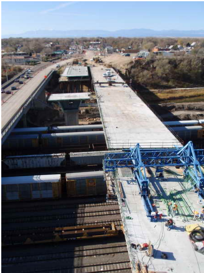
Figure 7 – Cantilever 4 WB Segmental Construction – November 4, 2009: Cantilever 4 WB (right) construction nears completion as it approaches the previously completed Cantilever 3 WB in the main-span. Pier Table 3 EB (left) will receive the form travelers when Cantilever 4 WB is complete. Roadway work occurs in the far background.
