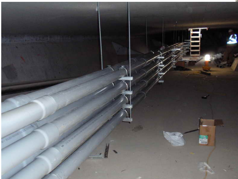
Figure 5 – Utility Work – October 28, 2009: The conduits are installed in Span 1 WB in preparation for Qwest Utilities (Telecommunications). Qwest will install their cables after Span 3 WB closure pour is complete.
