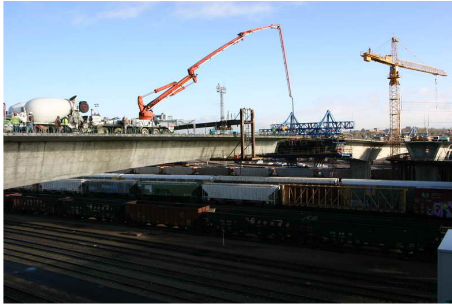
Figure 1 – Cantilever 4 WB Segmental Construction – October 22, 2009: A 52-m pump truck is staged on Cantilever 3 WB to facilitate concrete placement for Segment W4-7W.
