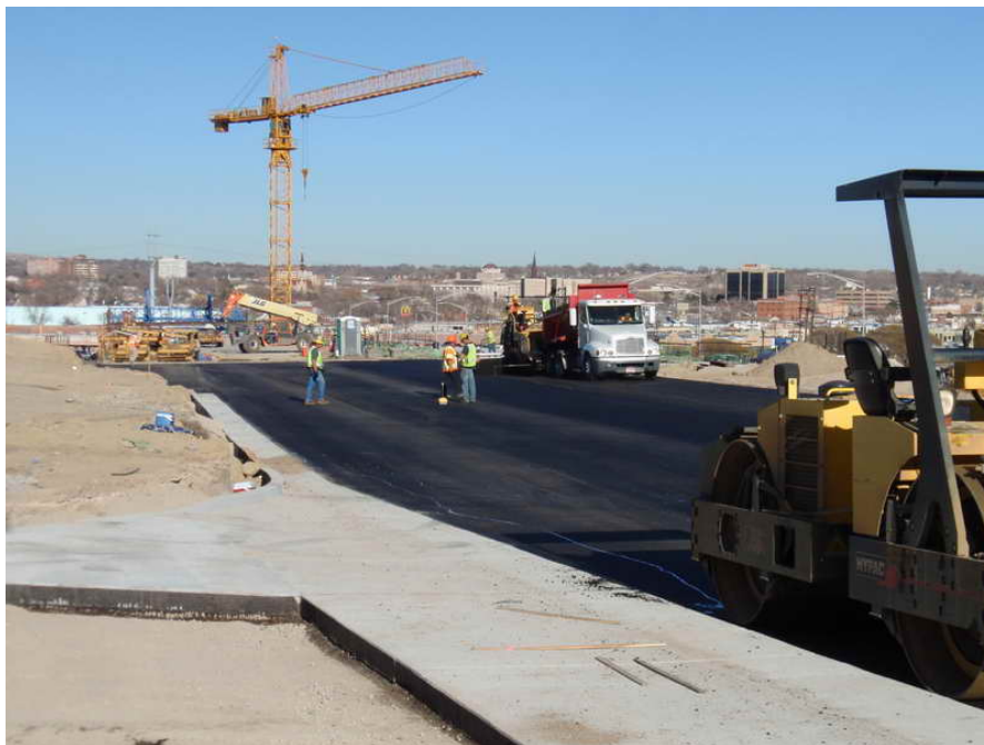
Figure 12 – West End Roadway Approach Construction – November 18, 2009: Paving operations take place for the approach on the westbound structure. All four lanes will be switched to the westbound bridge in early 2010.
