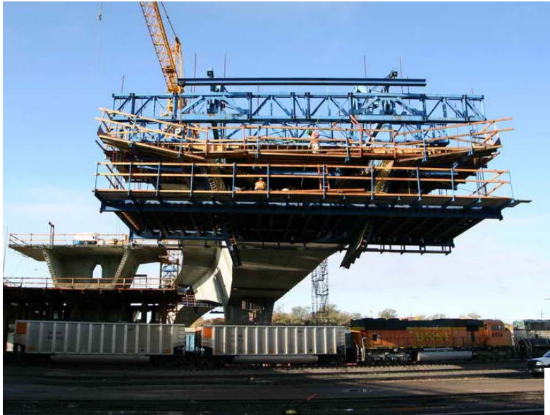
Figure 3 – Cantilever 4 WB Segmental Construction – October 22, 2009: A BNSF train passes under Cantilever 4 WB, as seen from below Span 5 WB. The form traveler is in position for Segment W4-7E.
