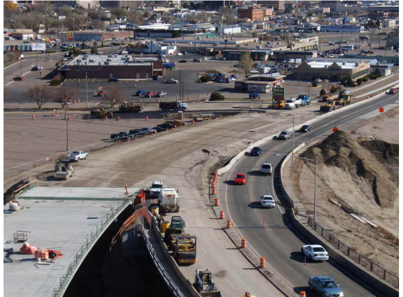
Figure 6 – East End Roadway Approach Construction – November 11, 2009: Paving begins at the entrance of the Midtown Shopping Center. The Contractor intends to complete paving operations before the winter season sets in.
