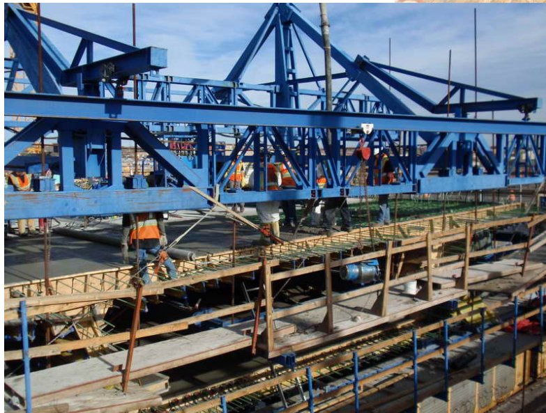
Figure 9 – Cantilever 4 WB Segmental Construction – November 6, 2009: The segment crew finishes the top slab for Segment W4-9W with the roller screed.
