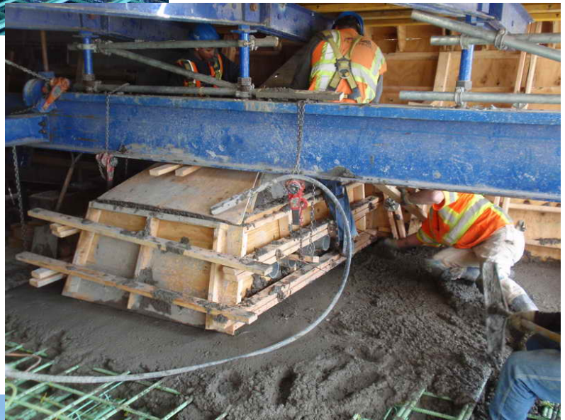
Figure 9 – Cantilever 3 EB Segmental Construction – March 12, 2010: Concrete is placed in the webs and deviator diaphragm and vibrated approximately two feet beyond the limits of the formwork. Once the diaphragm and web are completely filled, carpenters install plywood on the top of the deviators to help hold the hydrostatic pressure of the concrete. The remaining portion of the bottom slab is filled next.
