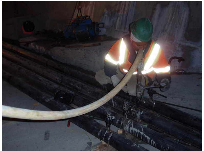
Figure 6 – Span 3 WB Grouting Operations – March 4, 2010: A Flatiron employee monitors the pressure of the grout as it is pumped into one of the draped tendons in Span 3 WB. The bottom slab tendons behind him were grouted after the draped tendons.
