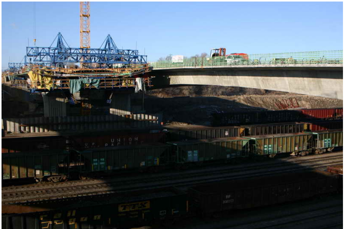
Figure 7 – Cantilever 3 EB Segmental Construction – March 5, 2010: Cantilever 3 EB construction continues over the UPRR tracks and the Arkansas River. These tracks are active during all operations, including concrete placement for the segments, maintaining no impact to the Railroad operations during construction.
