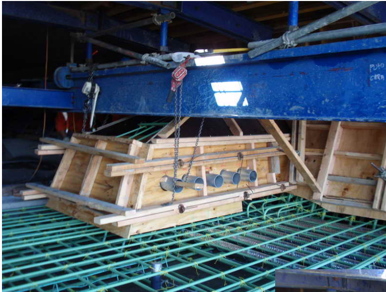
Figure 8 – Cantilever 3 EB Segmental Construction – March 9, 2010: Segment E3-8E deviator diaphragm forming, reinforcing, and post-tensioning installation is complete. The draped tendon rigid pipes in the deviator are rotated to a specific angle to maintain the tendon geometry upon installation and stressing after closure of the main-span. The core form support rail just clears the deviator.
