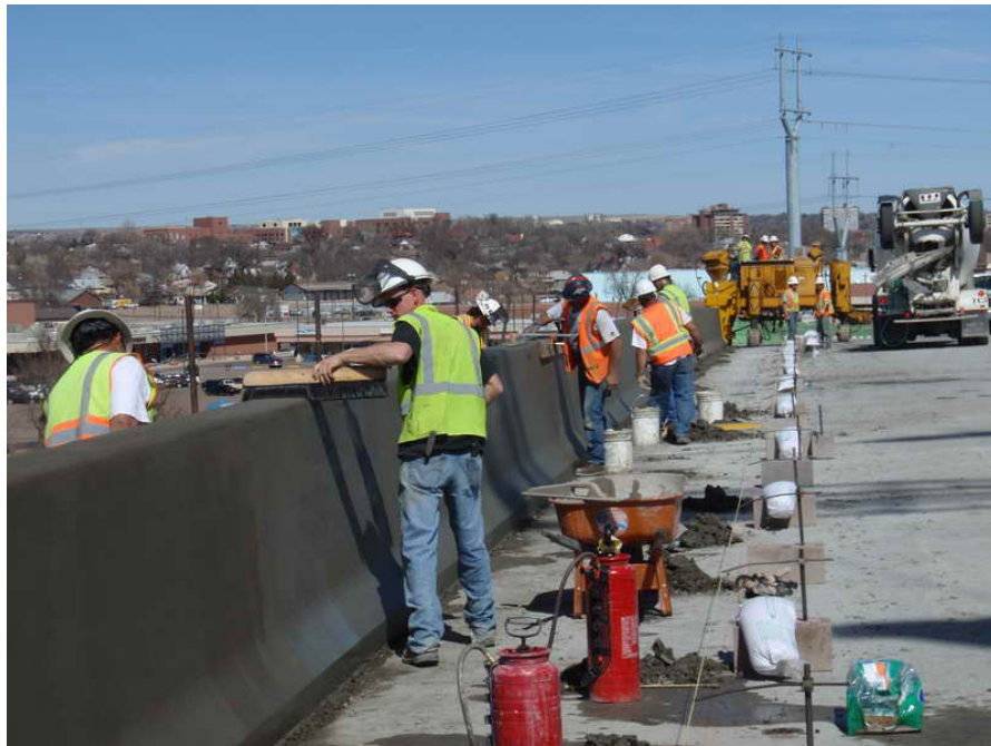
Figure 11 – WB North Barrier Construction – March 17, 2010: Workers finish and broom the surface of the 3'-10" tall north barrier behind the slip form machine.
