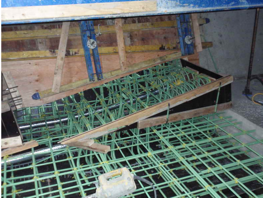
Figure 1 –Cantilever 3 EB Segmental Construction – February 19, 2010: Segment E3-6E contains two pair of double anchor blocks in the bottom slab. This photo shows how the typical interior web forms are adjusted by cutting the web channels to avoid the anchor blocks.
