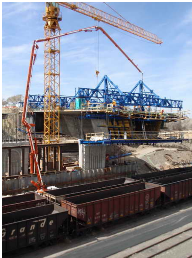
Figure 2 – Cantilever 3 WB Segmental Construction – March 18, 2009: The concrete pump is staged between the temporary shoring wall and empty UPRR coal train cars to place the concrete for Segment W3-2E.
