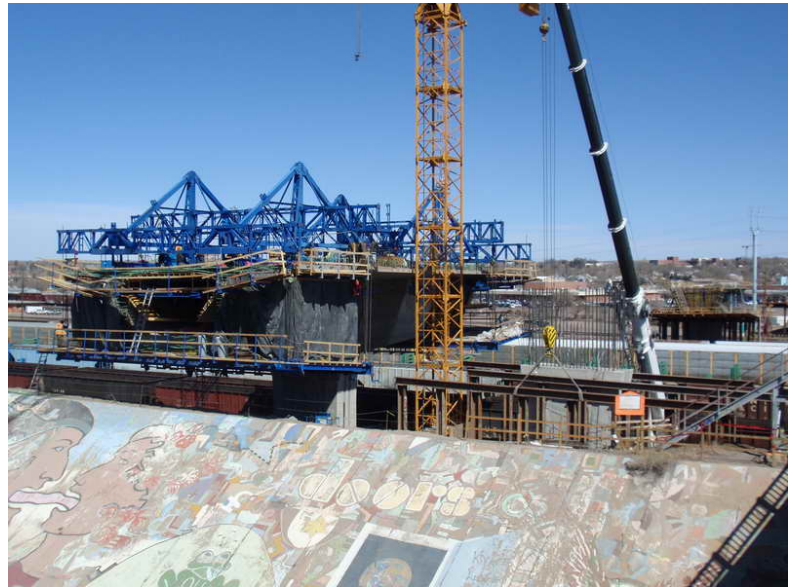
Figure 1 – Pier Table 3 EB Falsework Construction – March 11, 2009: Falsework bent erection begins at Pier Table 3 EB using a 175 ton crane behind the floodwall on the right, as work continues at Cantilever 3 WB, Segments W3-2W and W3-2E on the left.
