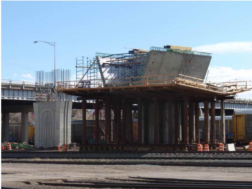
Figure 6 – Pier Table 4 WB Construction – March 31, 2009: With tension ties installed between the webs and the outside web forms stripped, Flatiron begins assembling the top slab formwork support scaffolding.
