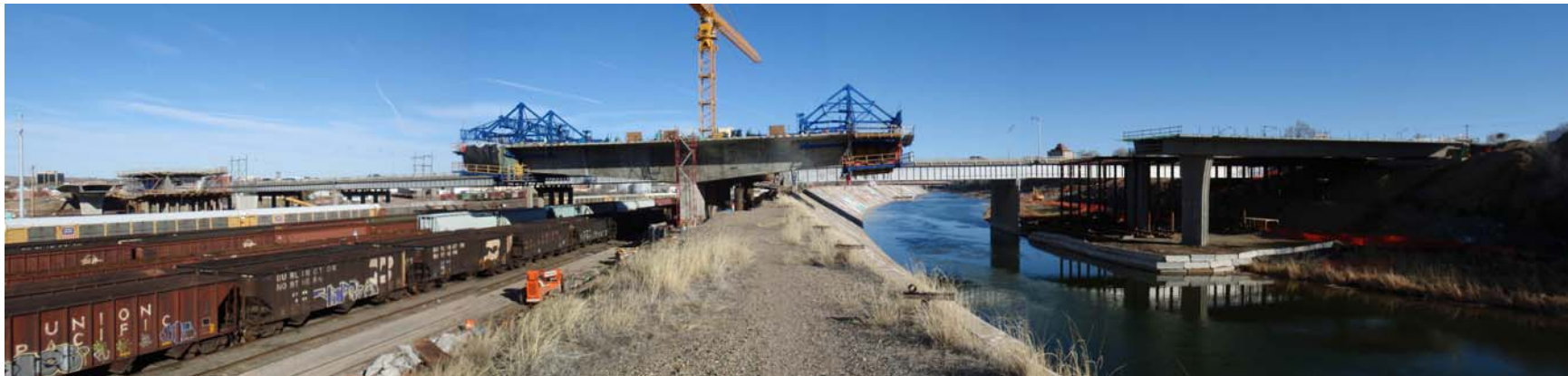
Figure 18 – Cantilever 3 WB Segmental Construction– April 13, 2009: A panoramic view of the project looking southeast from the top of the flood wall.
