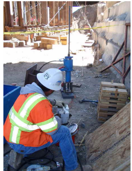
Figure 11 – Cantilever 3 WB Segmental Construction – April 6, 2009: A Flatiron employee tests the pull-out strength of a 1 1/4" diameter PT bar that was epoxied into the 5' diameter stability prop drilled shaft.
