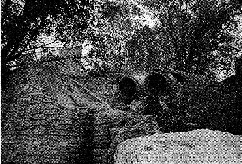
Figure 2.2. Broken sections of storm sewer pipe.
