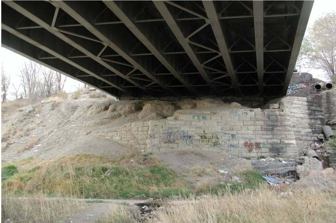
Figure 2.7 Erosion at West Abutment
