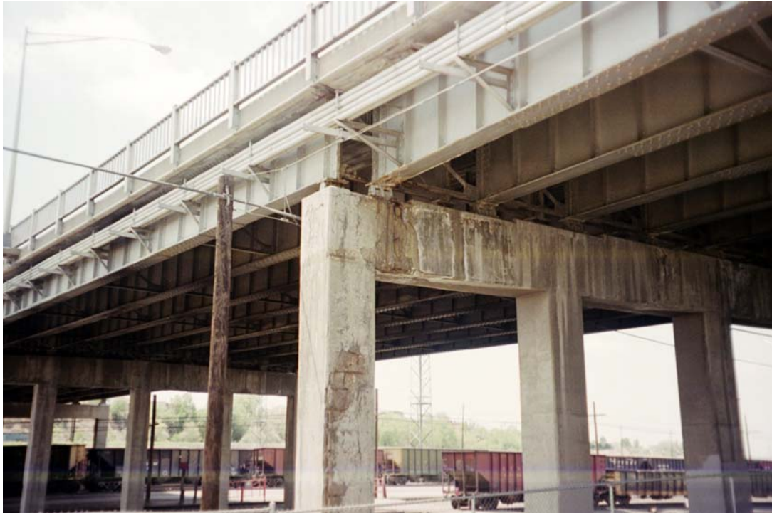
Figure 2.3 Bent 1 Concrete and Reinforcing Deterioration
