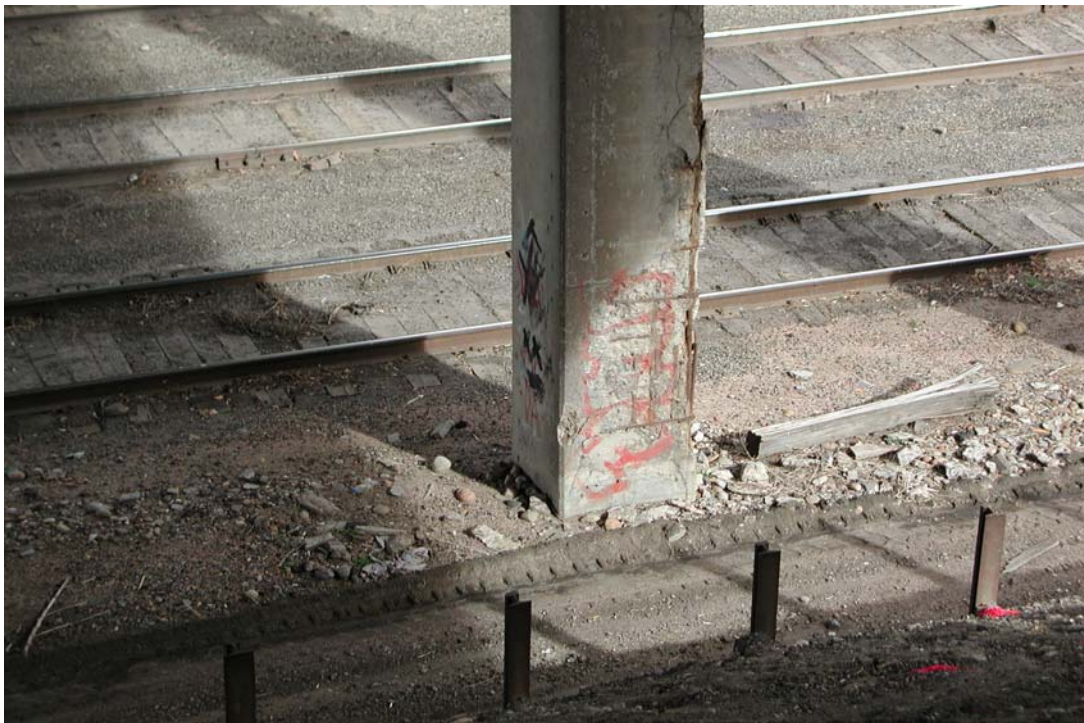
Figure 2.4 Bent 5 Concrete and Reinforcing Deterioration
