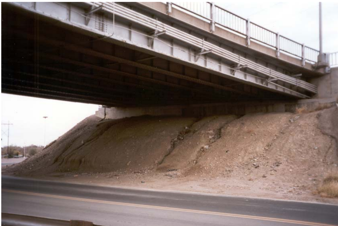
Figure 2.8 Erosion at East Abutment
