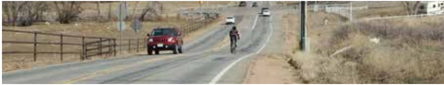
Insufficient shoulder width for multimodal use
