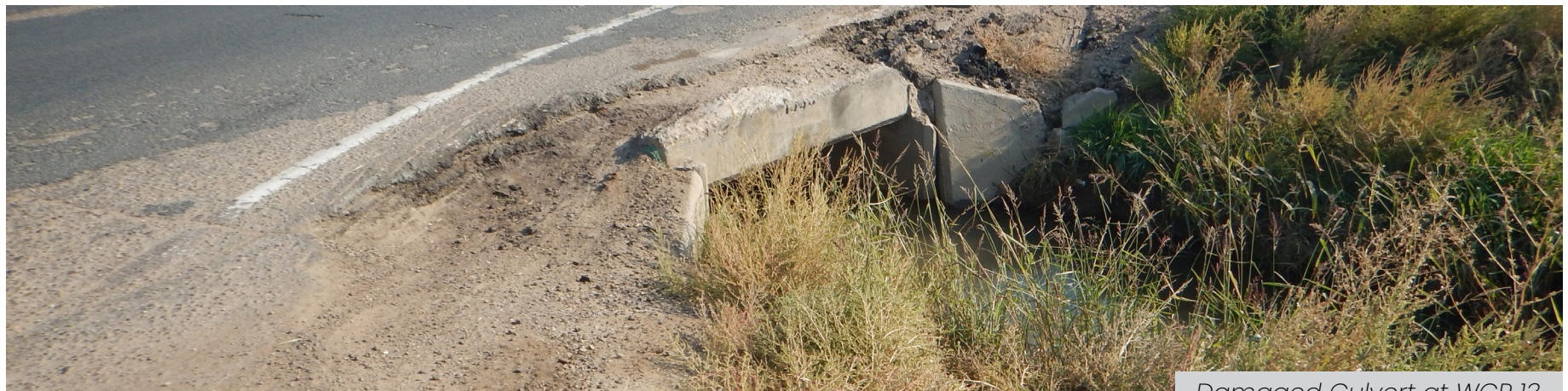
Damaged Culvert at WCR 13
