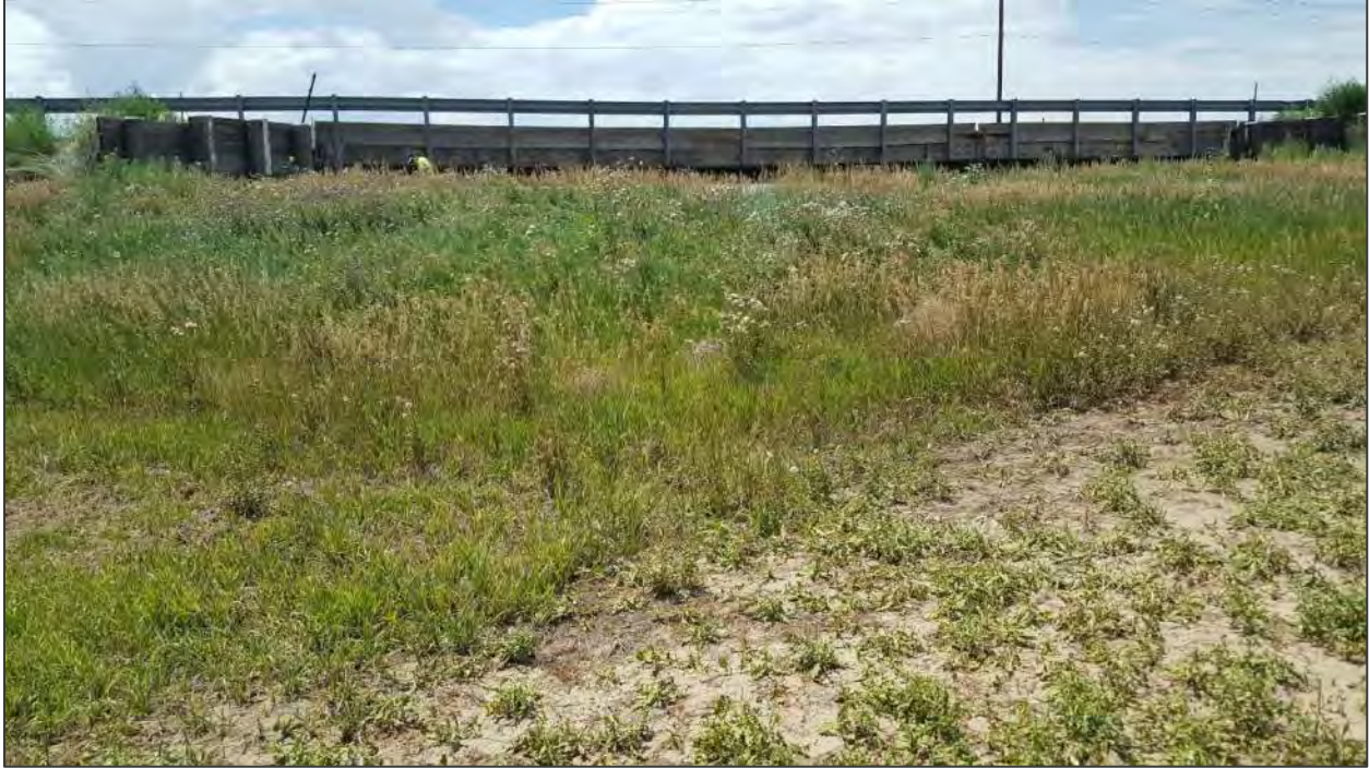
Figure 5. View looking at Bridge F-19-E and the high berm and drop to the swale channel downstream of the bridge.
