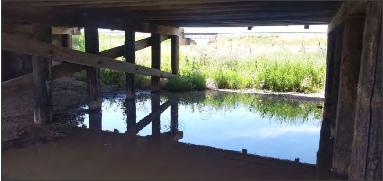
Figure 4. View looking upstream at shallow scour hole under US36 Bridge F-20-L.
