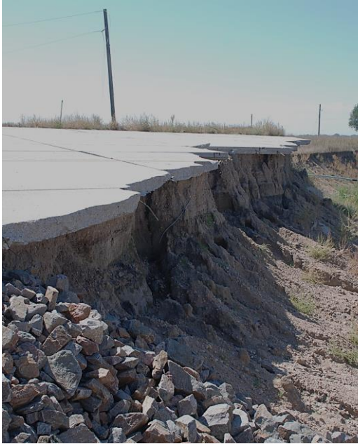
Damage to US 34 from the September 2013 flood event
