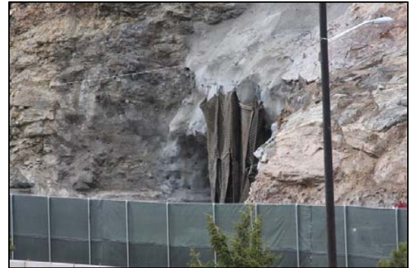
The use of blast mats and tall fencing along the highway help contain the blasts outside the tunnel to minimize the amount of rock that reaches the westbound lanes of I-70.
