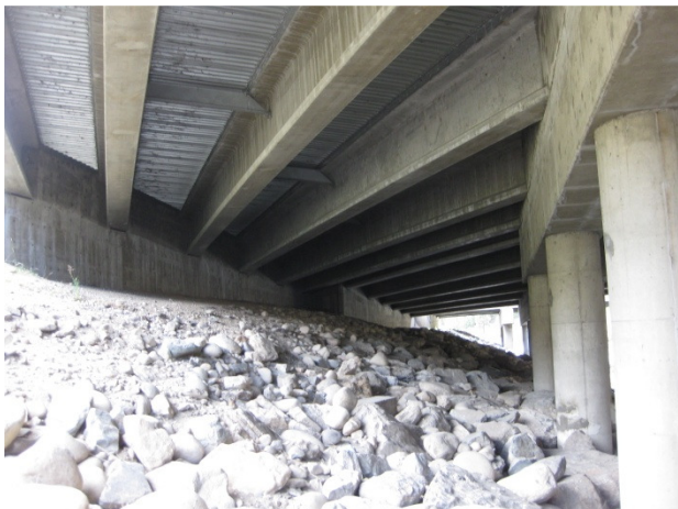
Figure 24. Efflorescence in pier cap
