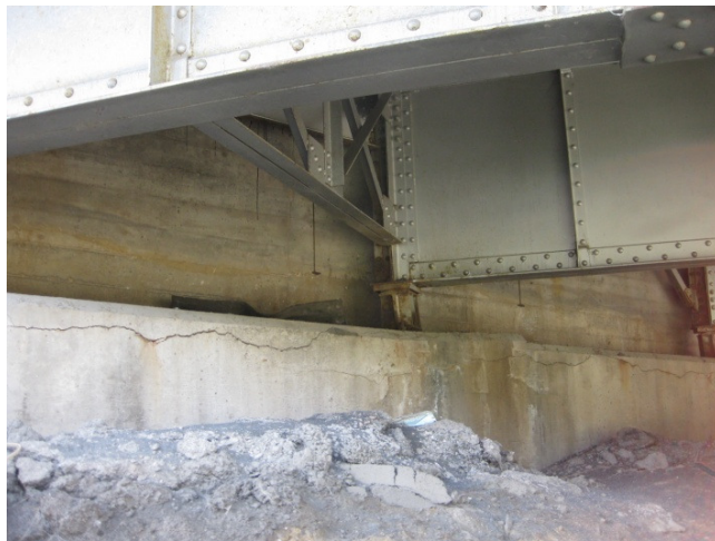
Figure 40. Cracks in south abutment
