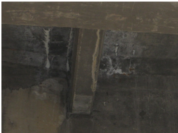
Figure 28. Efflorescence at deck bottom
