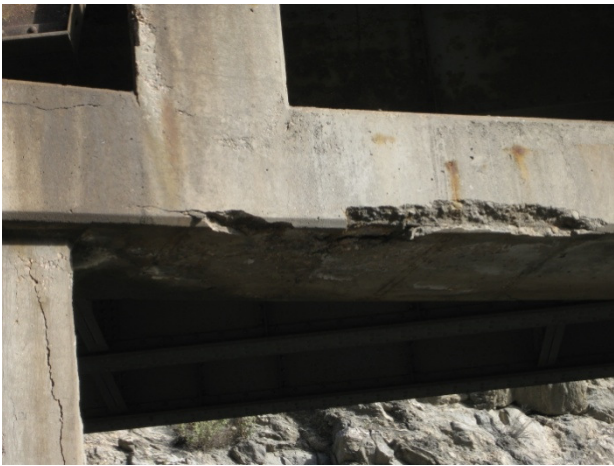
Figure 34. Cracks in pier cap and column
