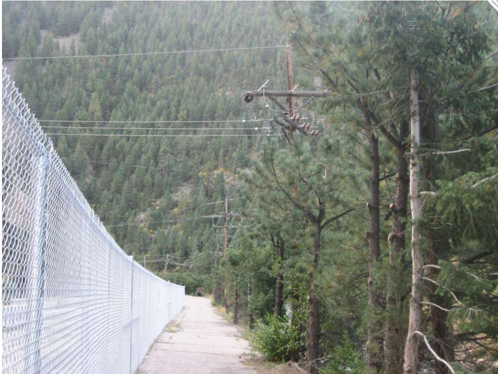
Figure 45. Overhead Xcel Energy electrical service lines with other utilities attached
