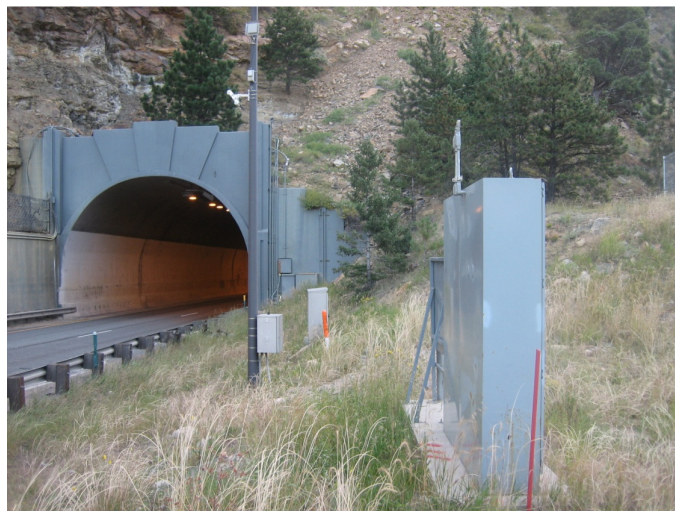
Figure 44. CDOT utility infrastructure at eastbound I-70 west tunnel portal
