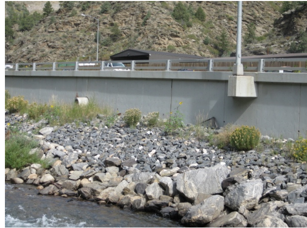
Figure 23. Light pole blister and RCP
