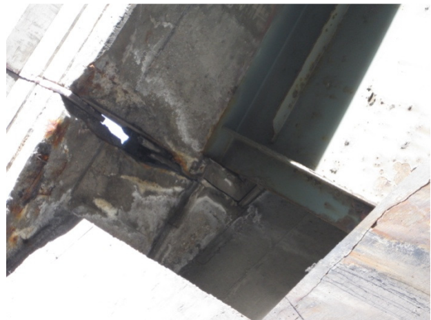
Figure 29. Corrosion around expansion joint
