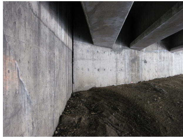
Figure 19. Offset in west abutment
