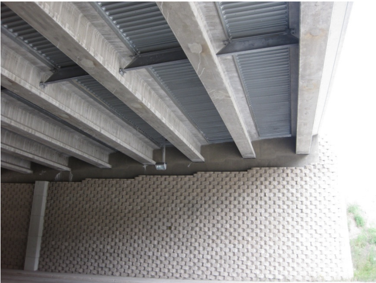
Figure 16. Some efflorescence in west abutment
