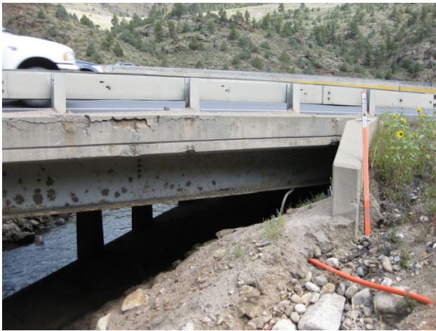
Figure 10. Cracks in deck near east abutment
