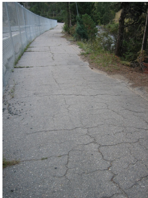
Figure 51. Bikeway cracked pavement
