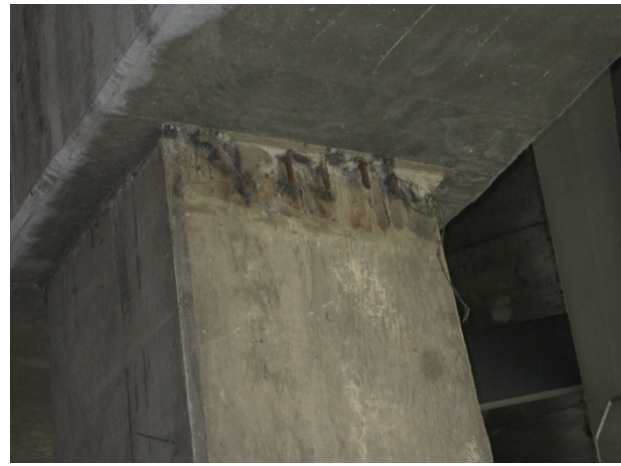
Figure 8. Exposed rebar in pier cap
