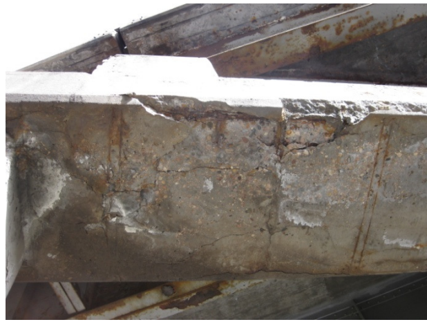
Figure 35. Exposed rebar below pier cap
