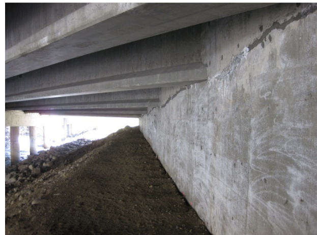
Figure 25. Efflorescence in abutment
