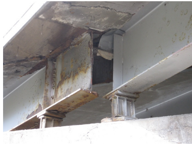
Figure 11. Rust in steel girders
