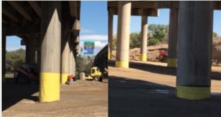
Photos showing progress of dirt build-up underneath I-25.
