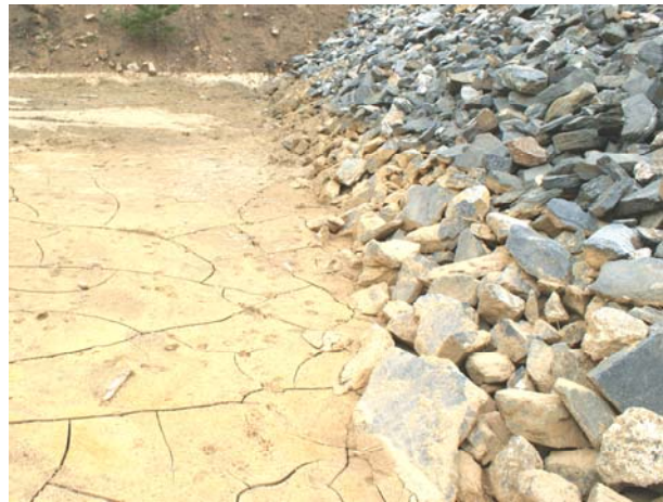
Mud on the face of this dam shows how these structures protect water quality by trapping sediment.
