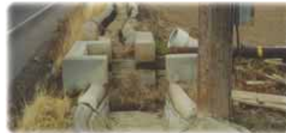
Existing Irrigation Issues along US 50
