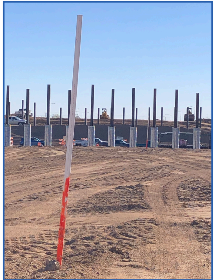
This photo shows a ground settlement monitor in the foreground, and 32 bridge piling foundations for the east and west abutments for the bridge that will be constructed over Purcell Boulevard.
