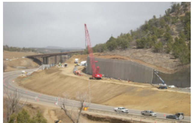
US 160 is widened to four lanes (with construction of a second westbound lane)
