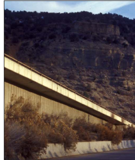
A | Where possible, allow for landscape screening to buffer the view of retaining walls.
