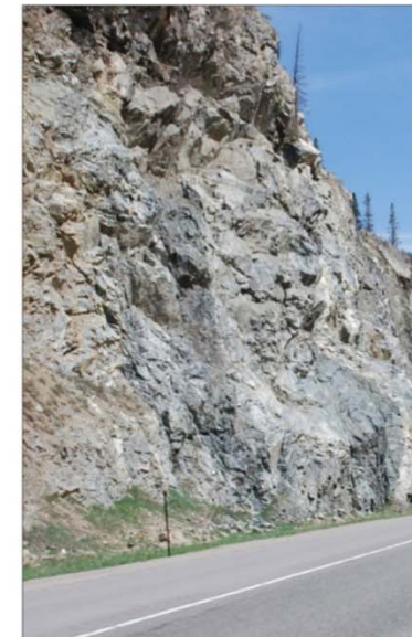
D | Color staining techniques will blend new rock cut with existing rock features.
