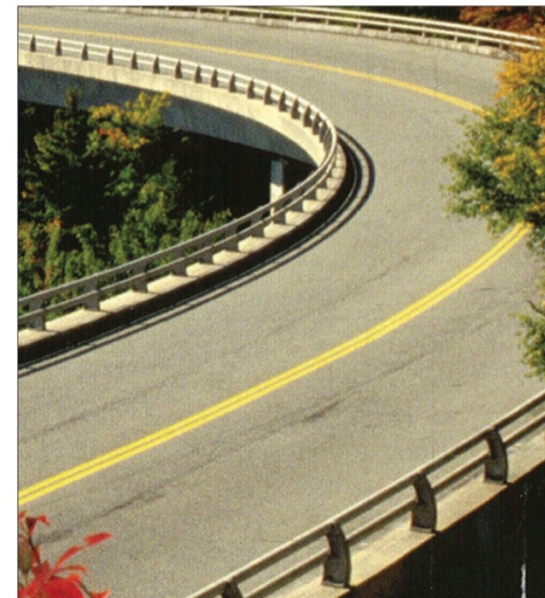
C | Utilizing attached metal rails on bridges rather than concrete barriers adds to the transparency and thin appearance of the span.
