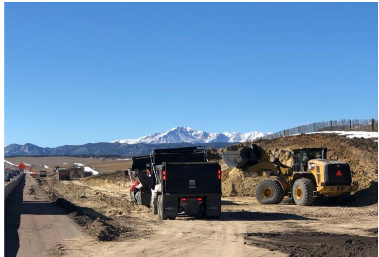
Crews began excavation measures on the shoulders of I-25 in the southern section of the project.
