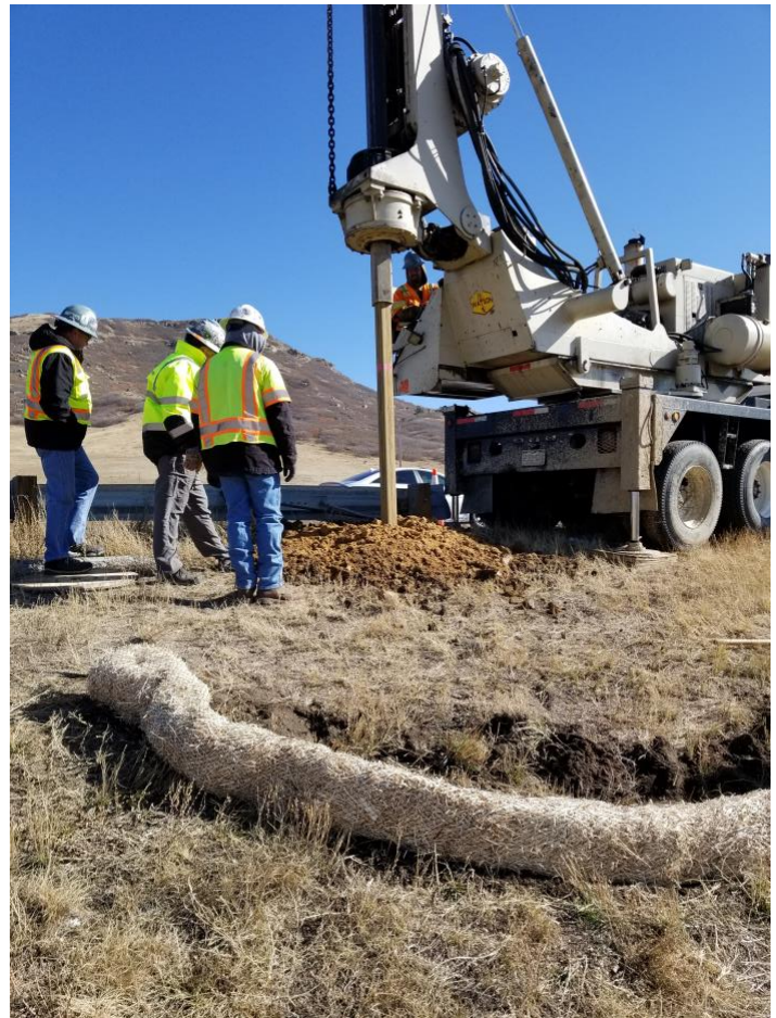
Workers run a drill rig while testing a location for a future caisson.
