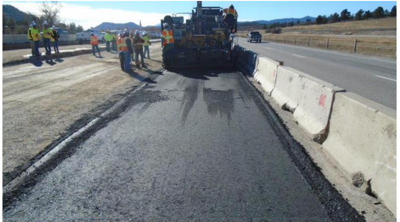
Crews began paving in the center median of I-25 between Plum Creek Parkway and Sky View Lane. Once completed, the entire corridor will have new asphalt pavement.
