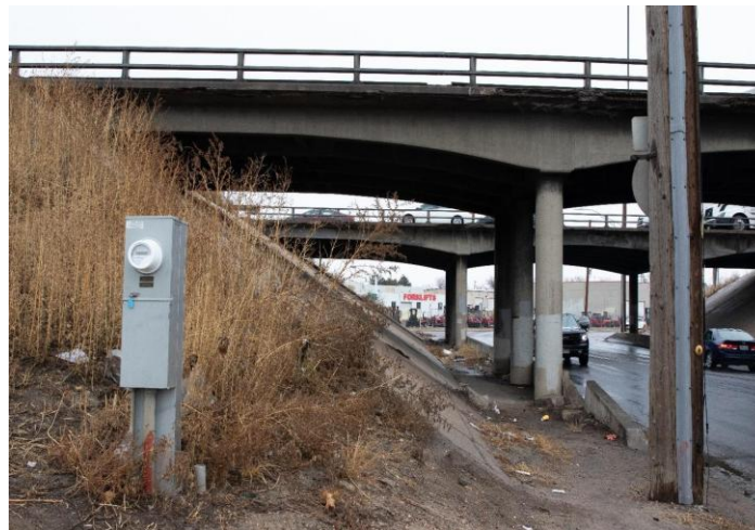
Figure 1-7. Substandard Bicycle and Pedestrian Crossing Under I-270
