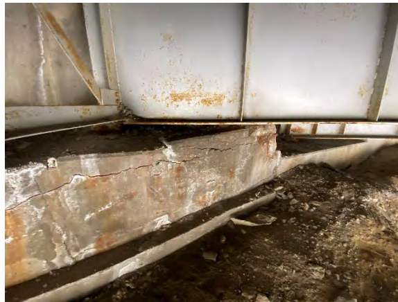
Figure 17. Delamination, rust staining, and failed patch at right end of Abutment 4
