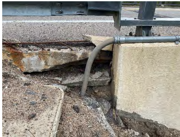
Figure 49. Typical undermining of approach slabs and damage to curbs on approach slabs. Right side of rear approach slab
