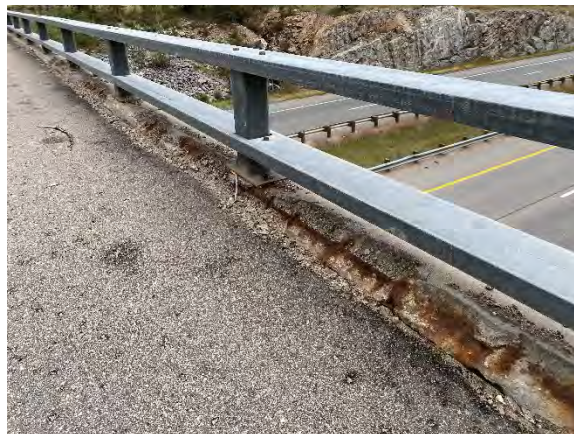
Figure 47. Typical spalls with exposed corroded reinforcement in curbs and “Type N” bridge rail
