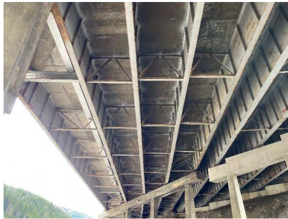
Figure 12. Typical view of underside of deck showing areas of patch and cracking with efflorescence
