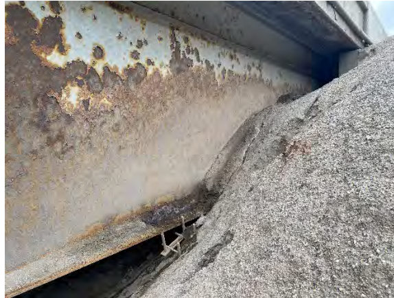
Figure 13. Debris on Girder 1A with uncovered area
