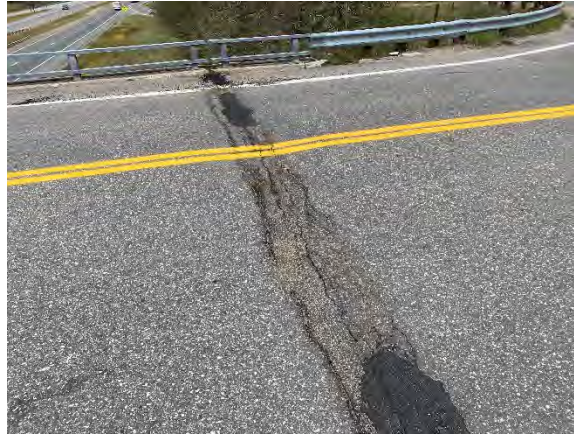
Figure 48. Transverse cracking of asphalt over compression joint at Abutment 3
