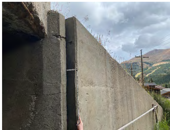
Figure 61. Leaning of southeast wingwall
