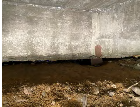
Figure 36. Off-center pile under Girder C at Abutment 1
