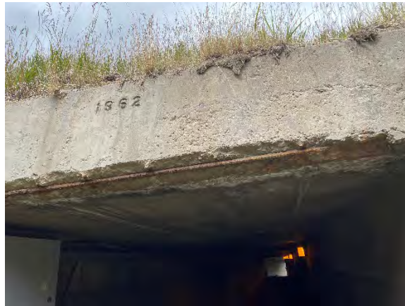
Figure 60. Spall with exposed rebar at outlet
