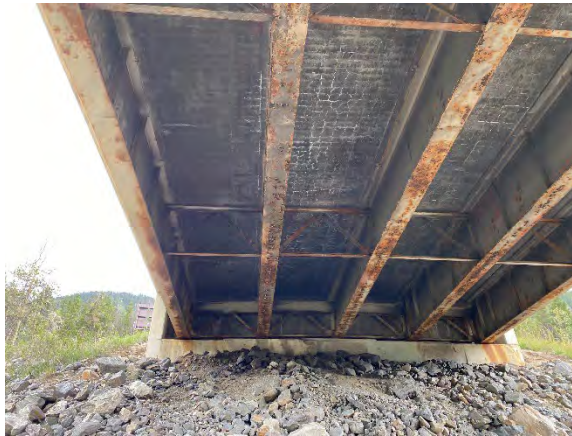
Figure 50. Typical view of underside of deck showing areas of cracking with efflorescence, Span 2 at Abutment 3
