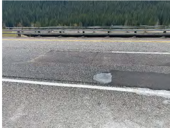
Figure 39. Asphalt patches in wearing surface
