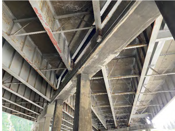
Figure 18. Failing, cracked patches on bottom edges of Pier 3
