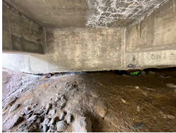
Figure 35. Exposed piles at Abutment 1
