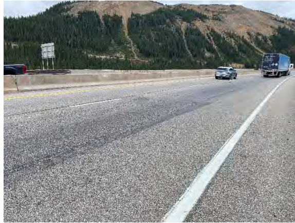
Figure 7. Asphalt patches in wearing surface.
