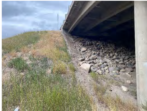
Figure 37. Erosion of berm embankments
