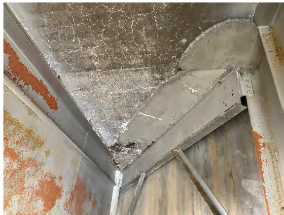
Figure 25. Cracking with efflorescence on underside of joint header at Abutment 4
