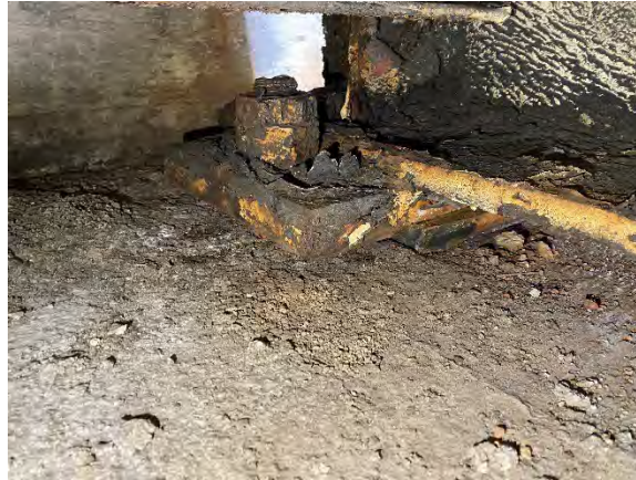
Figure 52. Crushing and bulging of bearing pad 3E
