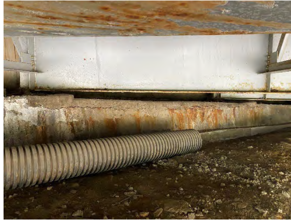
Figure 16. Delamination and rust staining on Abutment 1 girder seat
