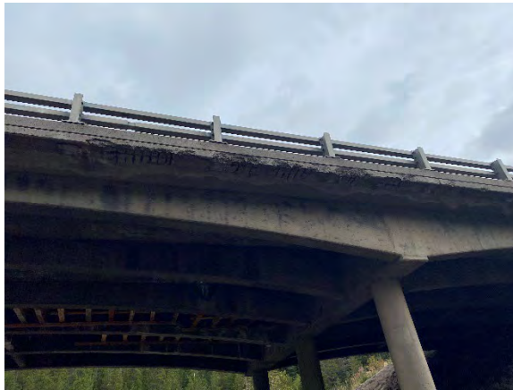
Figure 45. Typical spalling with exposed corroded reinforcement at edges of the deck
