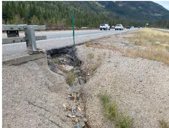
Figure 30. Erosion holes at ends of approach curbs
