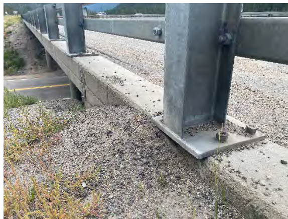
Figure 40. Disengaged nuts on bridge rail anchors
