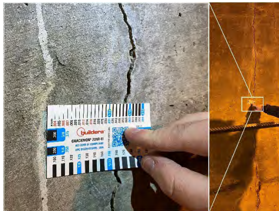
Figure 58. Typical wide width circumferential crack in culvert barrel
