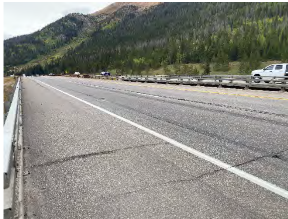
Figure 29. Asphalt rutting in driving lane
