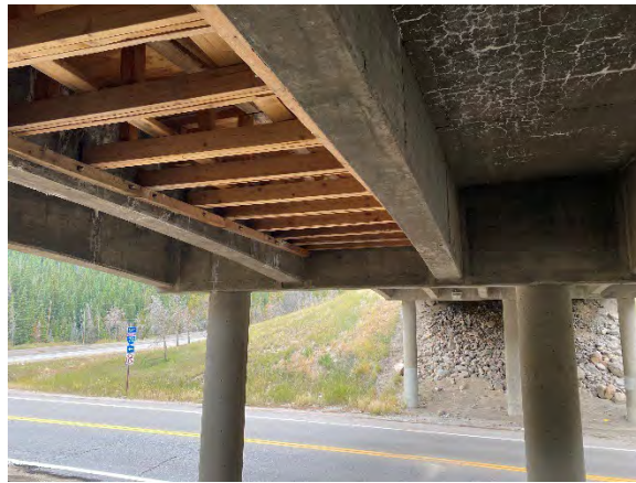
Figure 33. Permanent form work for concrete repair (Bay 3D) and map cracking with efflorescence (Bay 3C)
