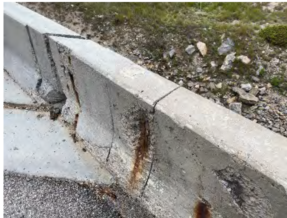
Figure 8. Typical deterioration of outside bridge rail
