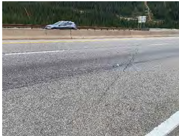
Figure 10. Transverse cracking of asphalt over Abutment 1
