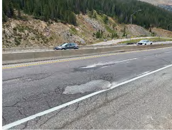
Figure 20. Typical potholes in asphalt wearing surface
