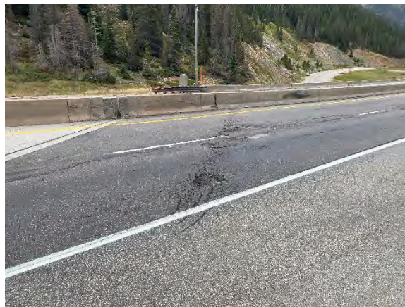
Figure 22. Transverse cracking in asphalt wearing surface over Abutment 1
