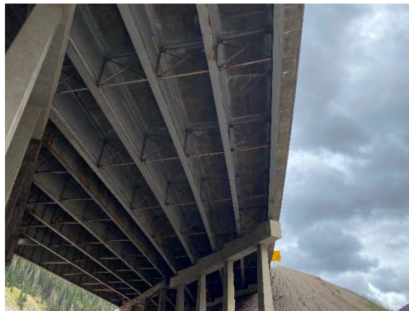
Figure 24. Typical view of underside of deck showing areas of cracking with efflorescence
