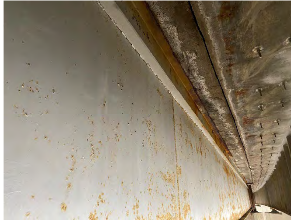
Figure 11. Drainage through longitudinal joint with F-13-P on to Girder E, corrosion on top flange of Girder E
