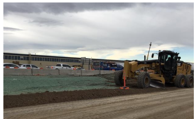
Covered dirt along Stapleton North Drive, December 2019
