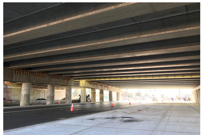
Peoria Street after 12-foot wide shared-use sidewalks are installed on the east side. The west side will have 8-foot wide walkways.
