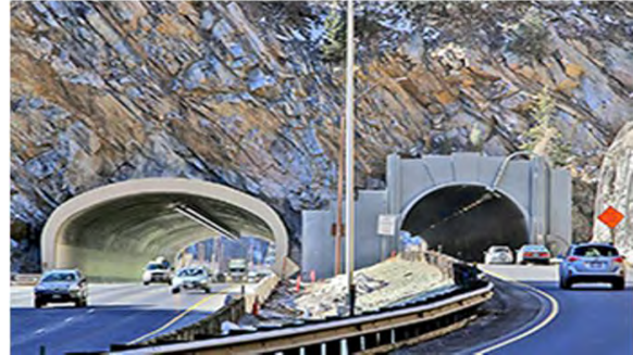
This photo from the Twin Tunnels on I-70 outside of Idaho Springs, Colorado, is an example of latest lighting technologies (on left) versus old standards of lighting.
