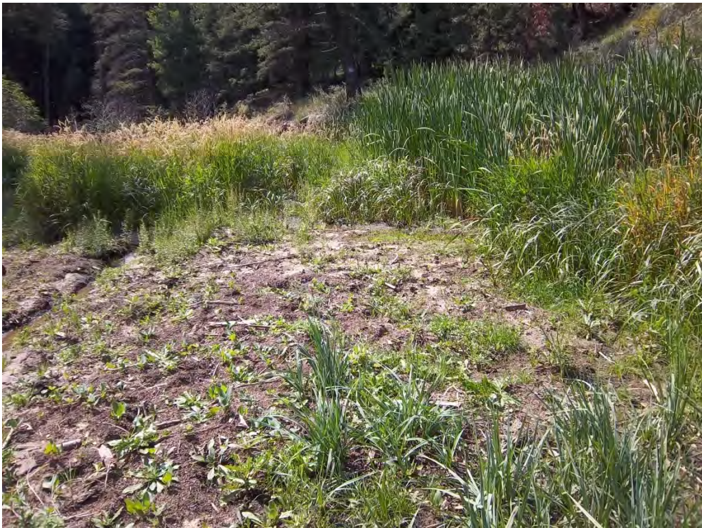
Photo Point 33: Wetland WL33 is formed where Johnson Gulch meets I-70 and backs up at a partially-blocked culvert, facing south.
