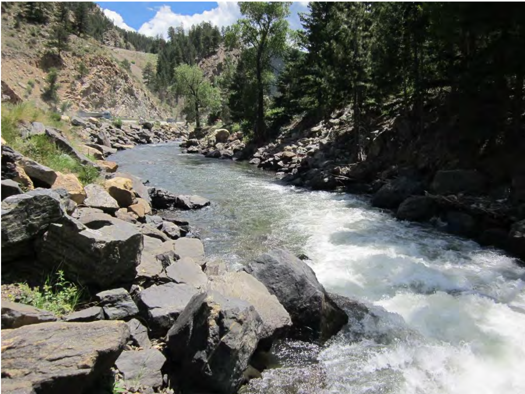
Photo Point 28: Facing downstream, both banks have been stabilized with rip rap.
