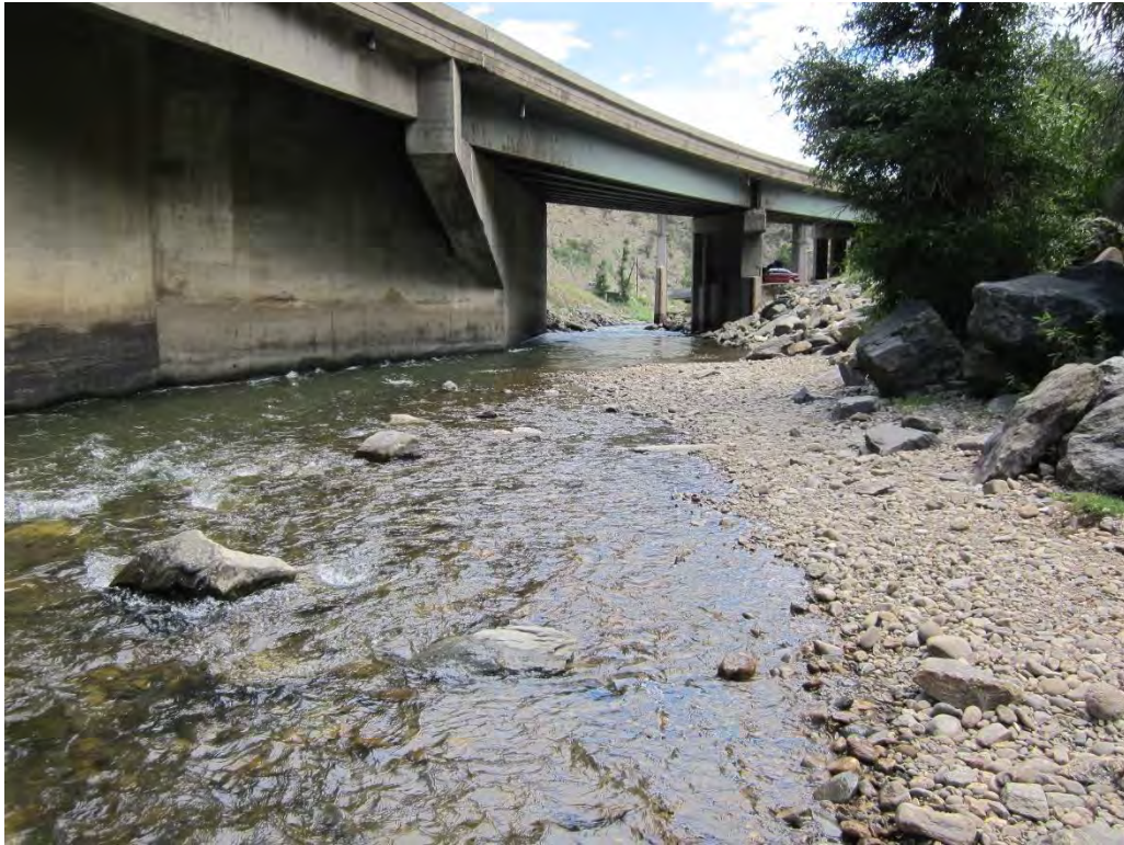
Photo Point 26: Clear Creek flowing under I-70, facing downstream. Flow is directed to the opening with concrete walls and rip rap.
