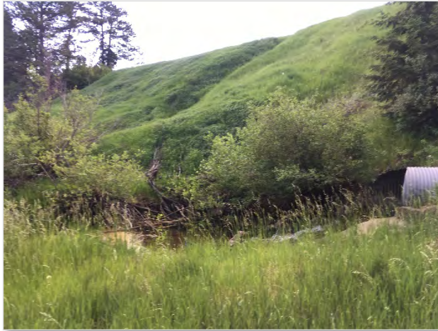
Photo 21. The downstream outlet of the Beaver Brook culvert under I-70 at the northeastern end of the Study Area, west of the Adams Acres property.
