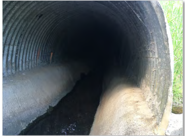
Photo 22. Looking inside of the Beaver Brook culvert under I-70. This culvert lacks natural sub-straight. While the top of the concrete is not designed as a formal rodent shelf, it can be used by various small wildlife species. Distance to inlet (~650 feet) with no lighting between acts as a barrier for wildlife to traverse.
