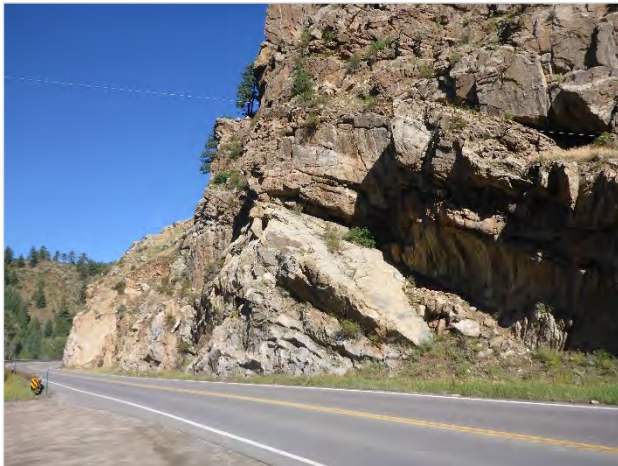
Photo 19. Picture looking west along the East Idaho Springs Road/I-70 Frontage Road, south of I-70 and the Veterans Memorial Tunnels near MP 242.3 during the Summer of 2017. This ridge is a large rock outcrop in the Project Corridor.
