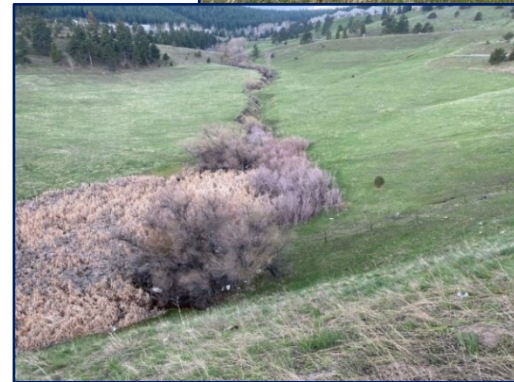
View below I-70, looking south from underpass at an unnamed drainage, east of MP 254.4
