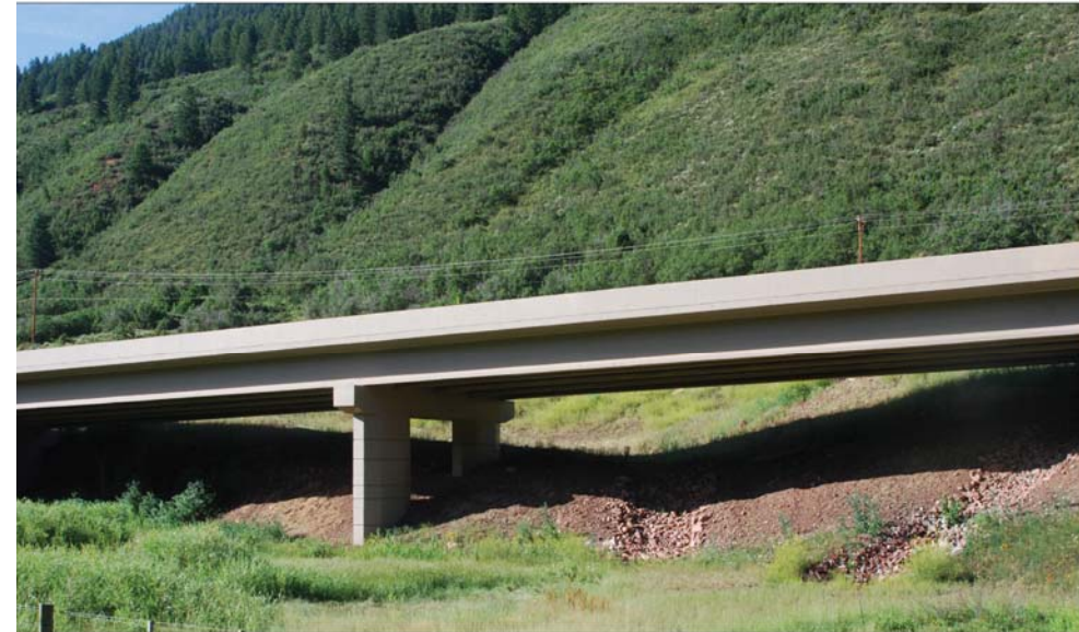
A | Roadway and bridge design should consider naturally occurring landforms and wildlife movement patterns.
