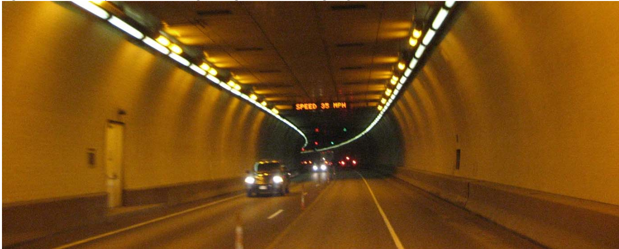
Figure 4. Reduced Speed Limit Message Using Variable Message Signs
