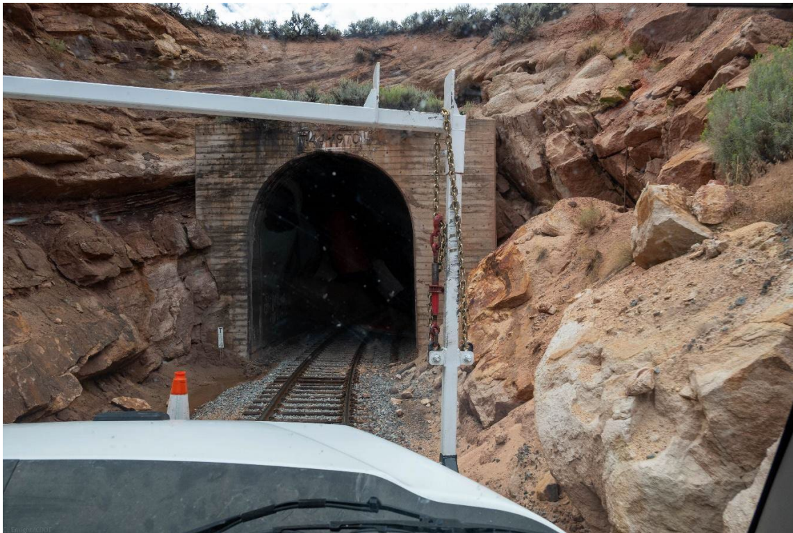
Figure 4: Existing Tunnel 44 with Probable Clearance Issue
