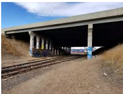
Right: Looking west at the BNSF Railway crossing over the South Platte River (directly west of the BNSF Railway crossing of I-25).
