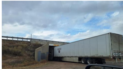
A truck attempting to drive through the box culvert.
