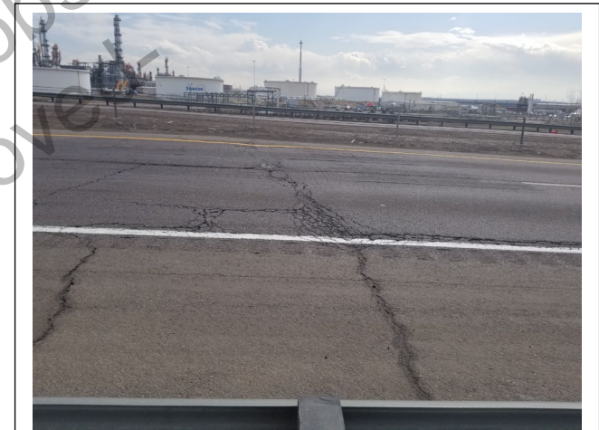
Figure 2-12. Example of Transverse Cracking and Deteriorating Pavement on I-270
