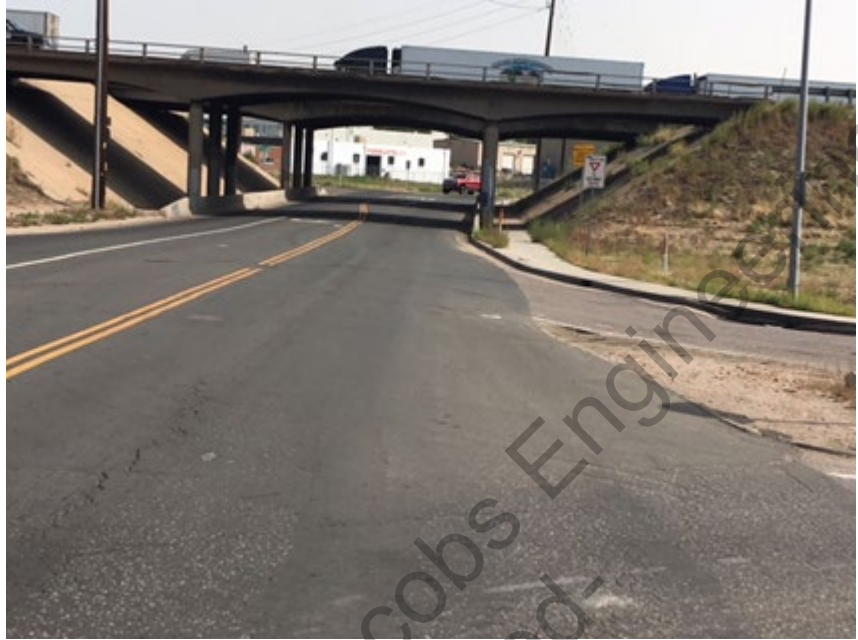
Figure 4-21. East 56 th Avenue East 56 th Avenue crossing I-270 looking north. Source: ACL Engineering
