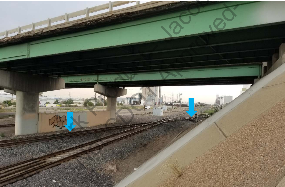
Figure 84. View of CB&Q/BNSF Segment 5AM.464.21 at I-270, indicated with blue arrows, view facing northwest. The segment is approximately 15 feet wide, which includes the tracks and a narrow strip of ballast on either side. The existing I-270 three-span bridge structures would be replaced with a single wider, two-span structure that spans the railroad right-of-way, and the current pier (pictured) would be removed.
