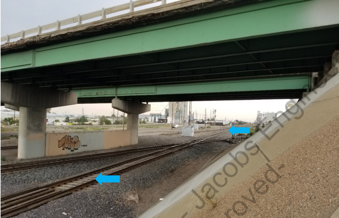
Figure 85. View of DP/UP Segment 5AM.472.41 at I-270, indicated with blue arrows, view facing northwest. The segment is approximately 15 feet wide, which includes the tracks and a narrow strip of ballast on either side. The existing two I-270 three-span bridge structures would be replaced with a wider, single two-span structure that spans the railroad right-of-way, and the current pier (pictured) would be removed. Jacobs, 2020.
