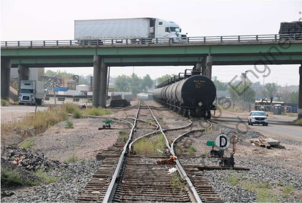
Figure 87. View of CB&Q/BNSF Segment 5AM.1298.3 at I-270, view facing south. The segment is 30 feet wide, which includes the double tracks and ballast on either side. The existing pair of three-span bridge structures would be replaced with a single wider, two-span structure that spans the railroad right-of-way.
