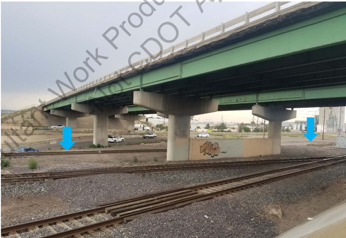
Figure 75. Location of UP Siding 5AM.4121.1 at I-270, indicated with blue arrows. View facing northwest. Jacobs, 2020.
