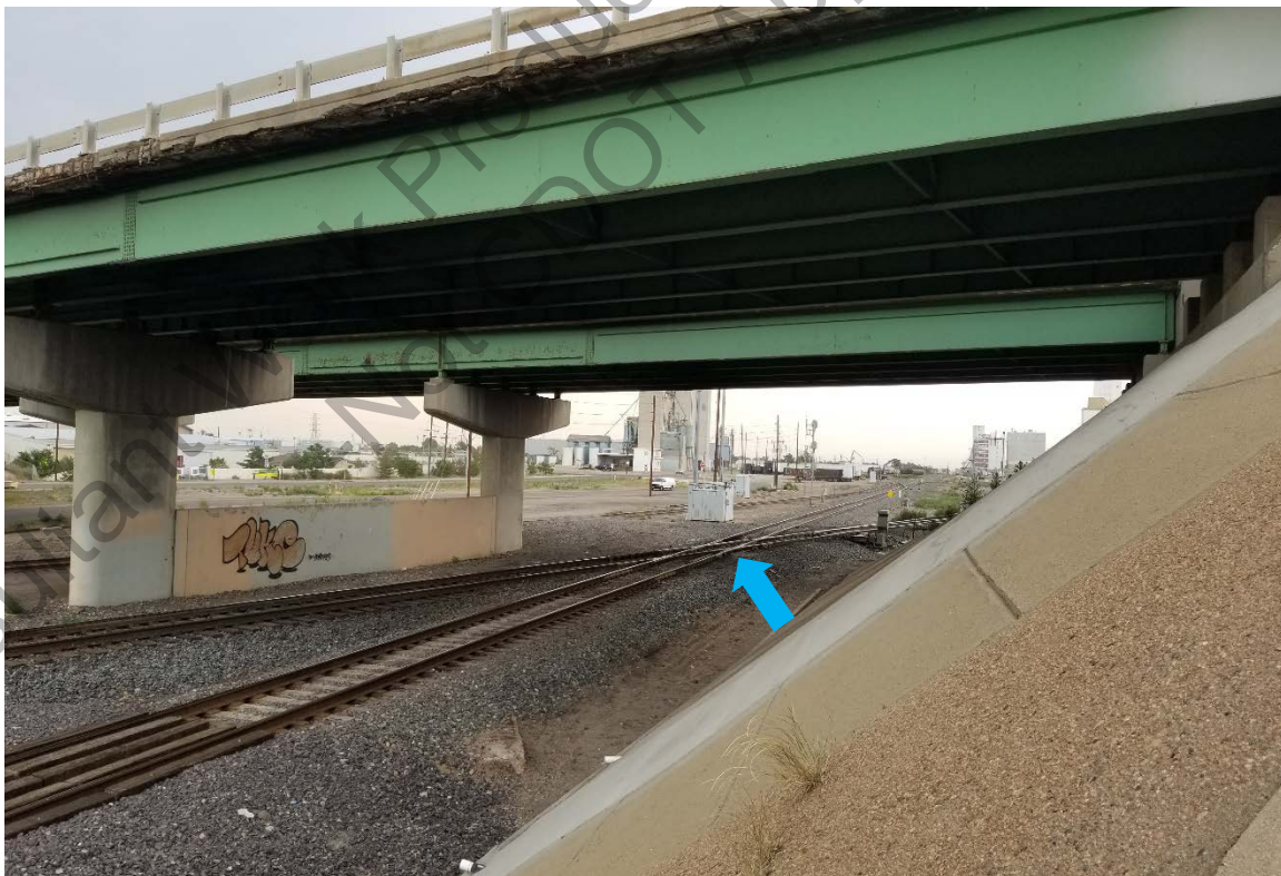
Figure 86. View of Sand Creek Junction beneath the westbound I-270 overpass, indicated with blue arrow, view facing north. The resource is approximately 20 feet wide, which includes the track junction and narrow strips of ballast on either side. The two existing three-span bridge structures would be
