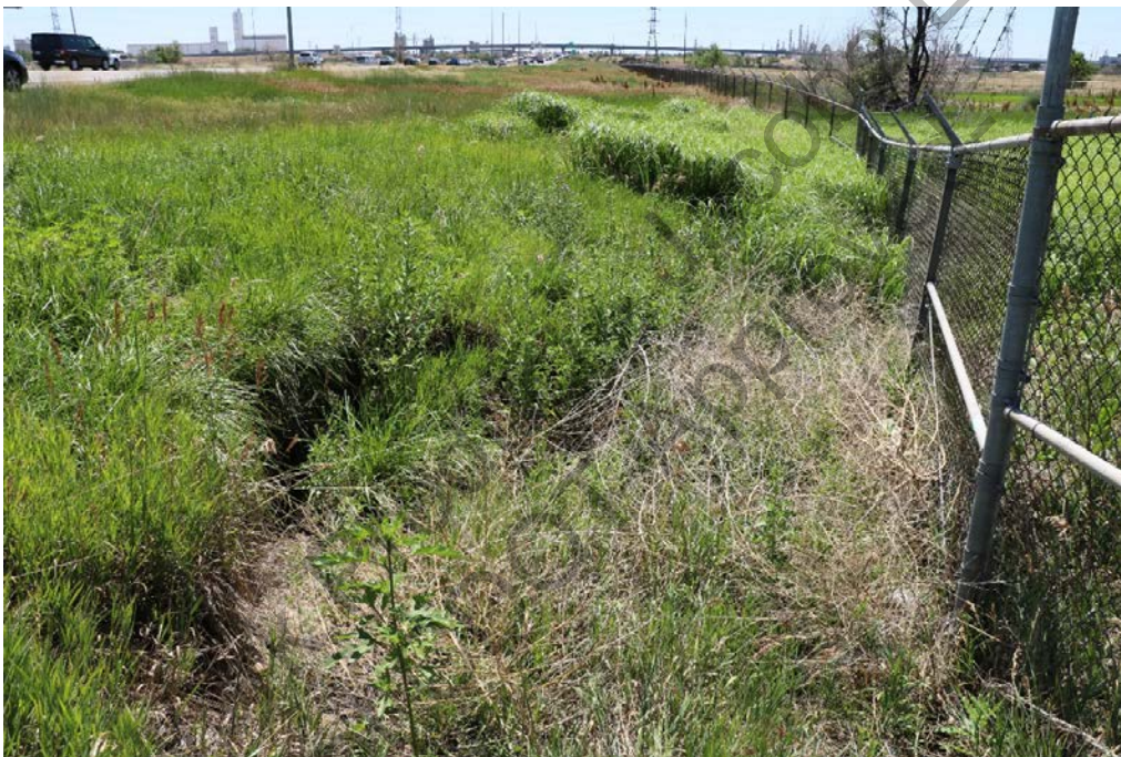
Figure 77. Location of the former Gardener's Ditch alignment at the south I-270 right-of-way, adjacent to the eastbound entrance ramp from York Street, view facing southeast. An underground drainage pipes would cross the location of the Gardener's Ditch north and south of the I-270 mainline and an above ground drainage would cross the ditch south of the I-270 mainline, within the right-of-way.
