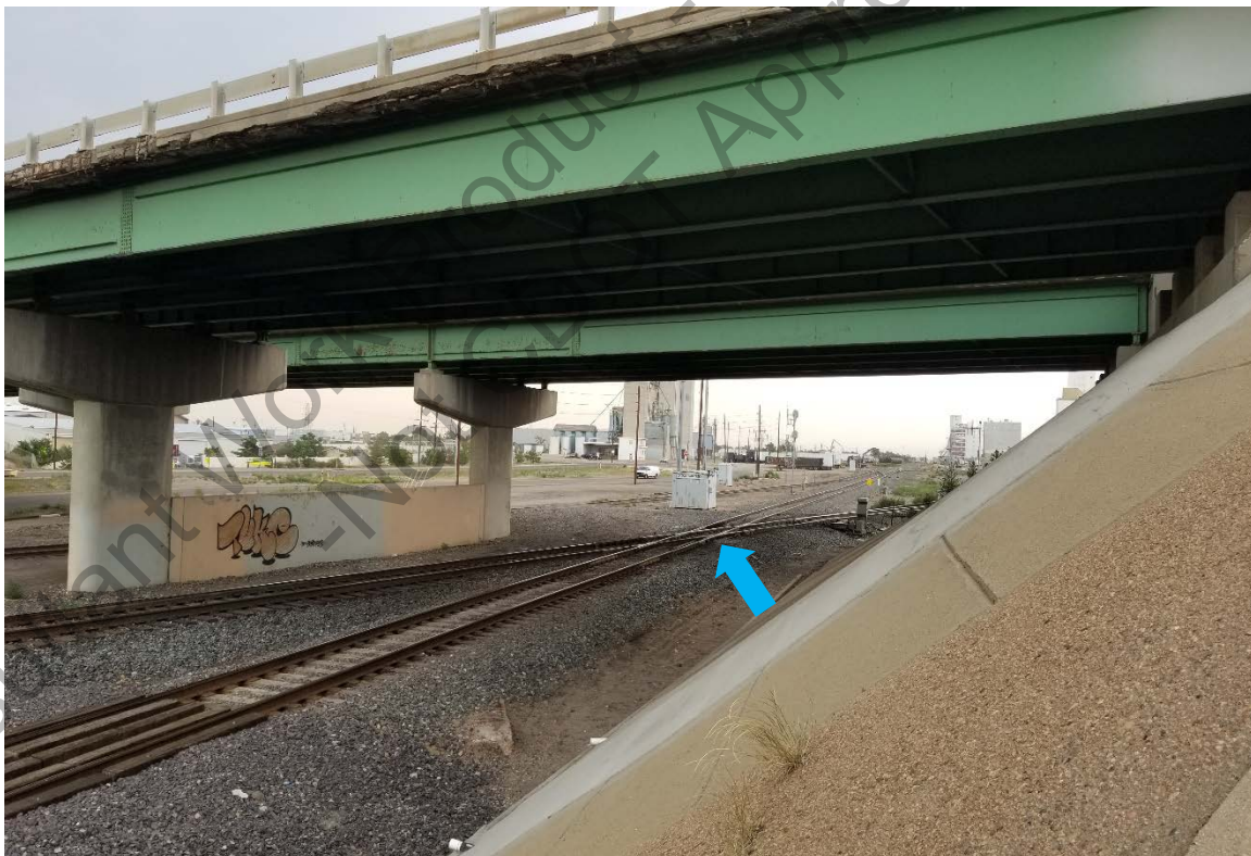
Figure 74. Location of Sand Creek Junction beneath the westbound I-270 overpass indicated with blue arrow. View facing north. Jacobs, 2020.
