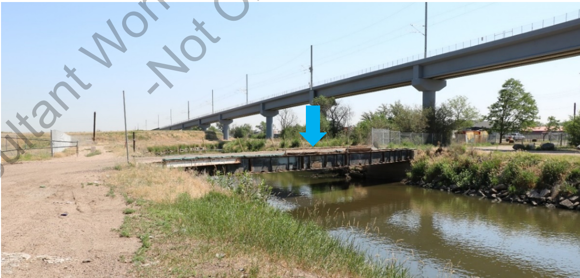
Figure 56. E 64 th Avenue bridge (5AM.4118) over the Burlington Ditch/O’Brien Canal. View facing northeast. Regional Transportation District North Metro (N line) elevated commuter rail line is visible to the east (right).
