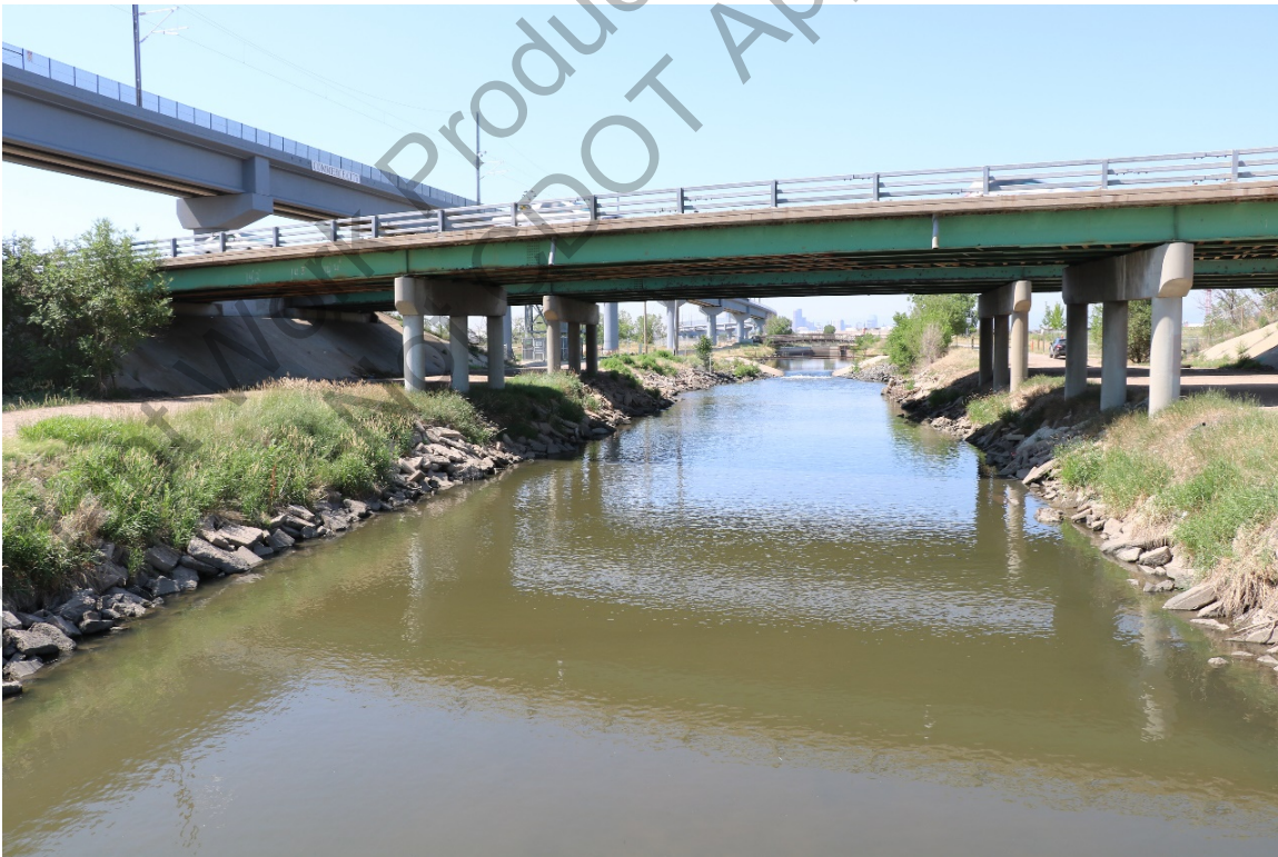
Figure 80. View of Burlington Ditch/O'Brien Canal at I-270, including elevated commuter rail line to the east (left), view facing south. The current I-270 bridges, which have bridge piers within the historic boundary, would be replaced with wider bridges that span the historic boundary with abutments outside of the boundary.
