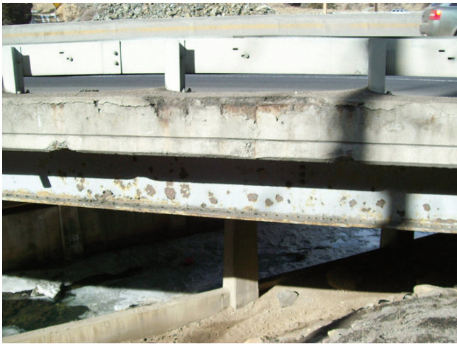
Lead-based paint on I-70 Hidden Valley Bridge over Clear Creek.
