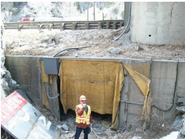
Box culvert under I-70, east of Twin Tunnels (looking south across I-70 toward Clear Creek).
