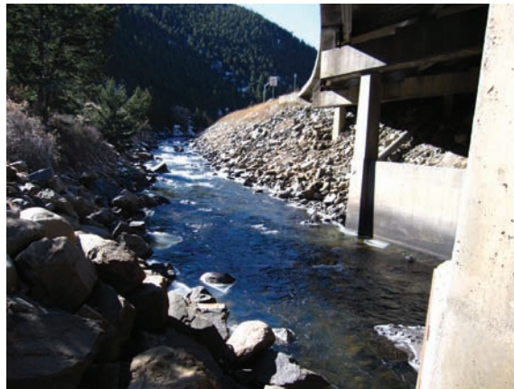
Clear Creek channel constriction/channelization.
