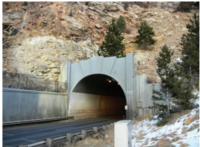
Zone of porphyritic rock above west portals. Note yellow staining on rock and retaining wall.
