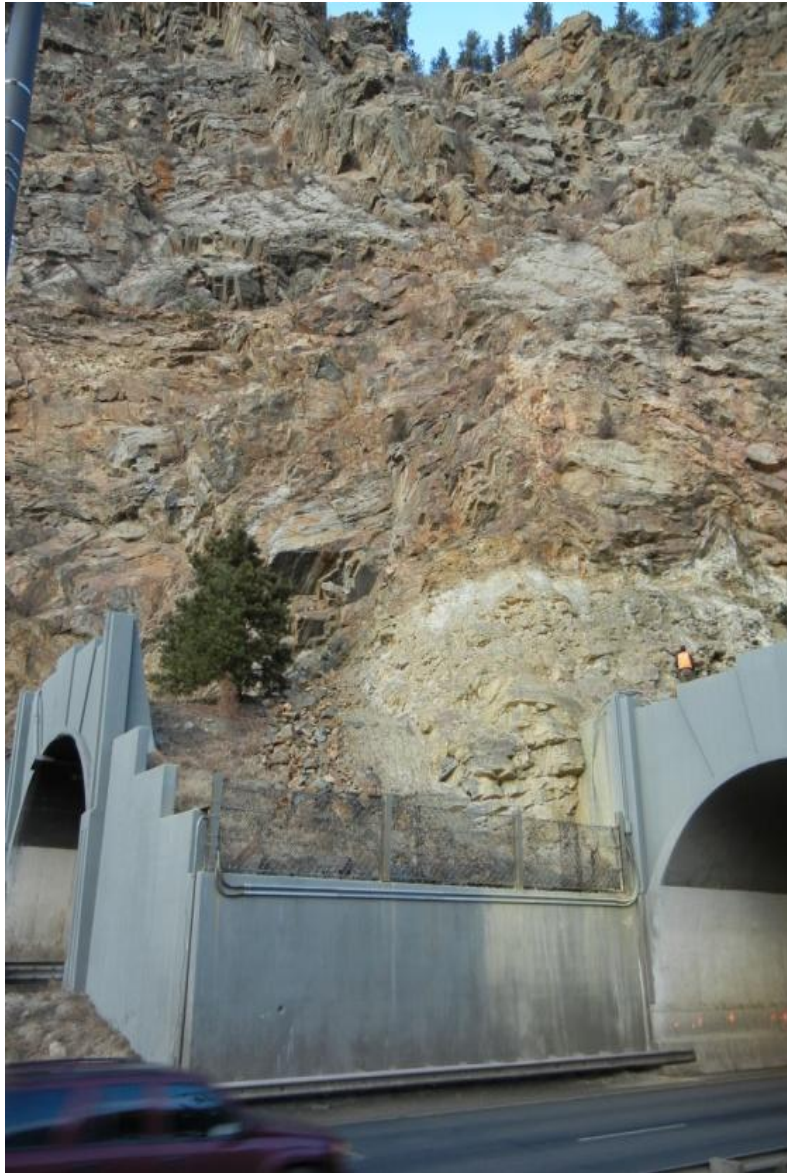
Figure 8. Rockfall Source Area and Rockfall at the West Portals.
