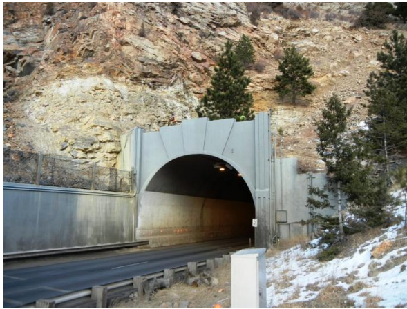
Figure 4. Zone of Porphyritic Rock above West Portals. Note Yellow Staining on Rock and Retaining Wall.
