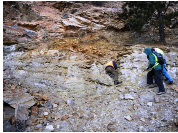
Figure 5. Zone of Poor Quality Rock above the West Portal of the EB Bore.
