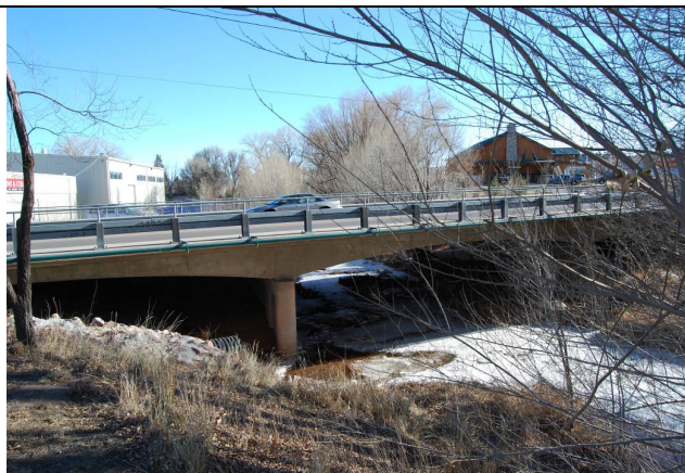
Figure 7. View looking southeast at US 24 along Fountain Creek from 21st Street. Photo from UTM 13, 512269 mE, 4299206 mN.
