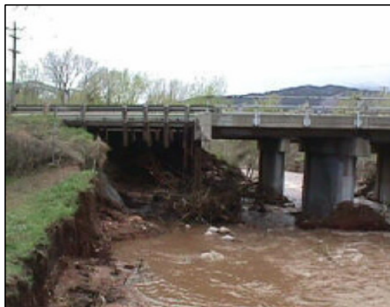
The US 24 bridge east of 21st Street was heavily damaged by flooding from a storm in 1999
