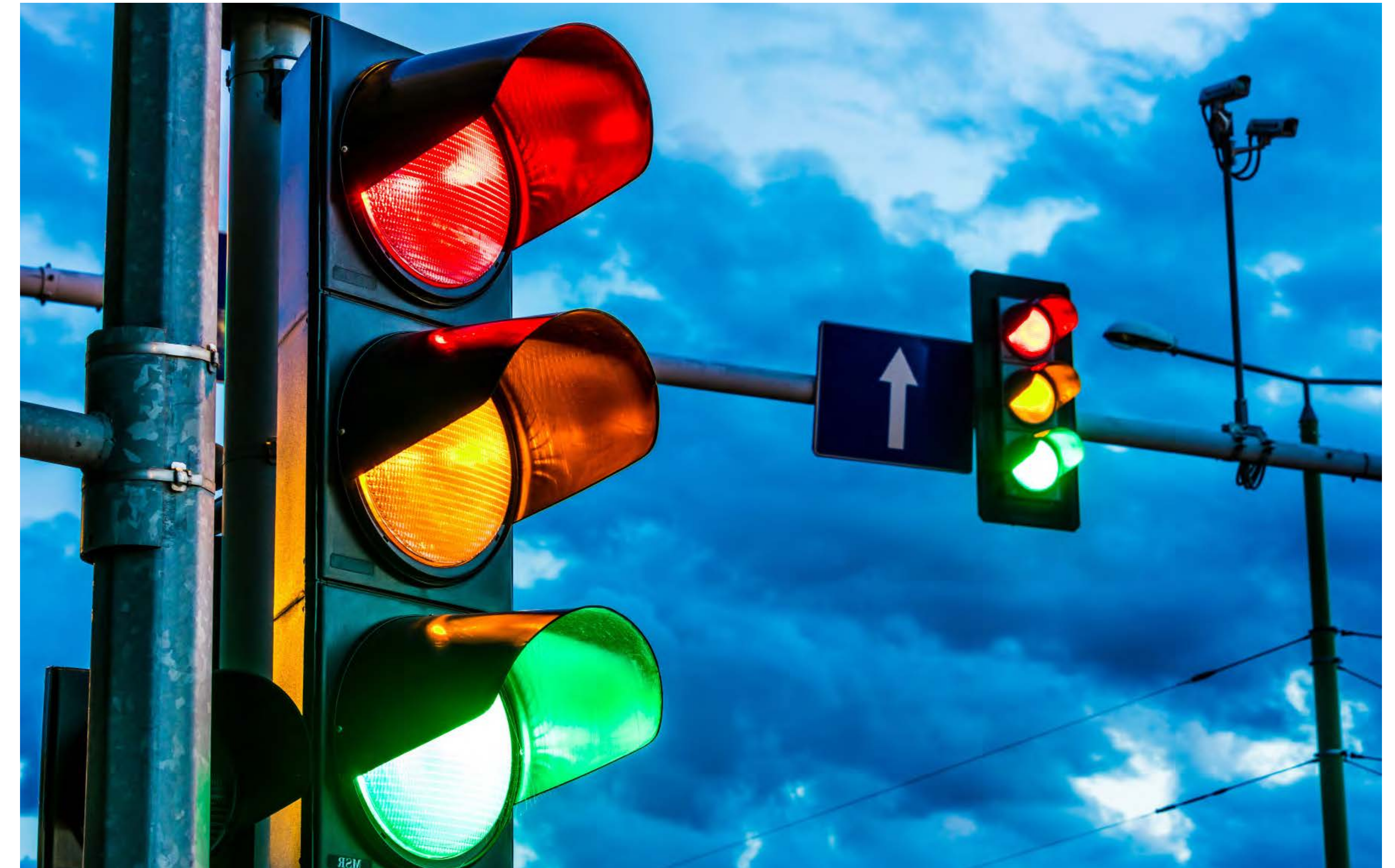
Traffic Signals on Street
