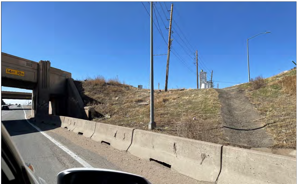
Photo 6: View of the railroad bridge and pedestrian walking area on Vasquez Boulevard facing south.
