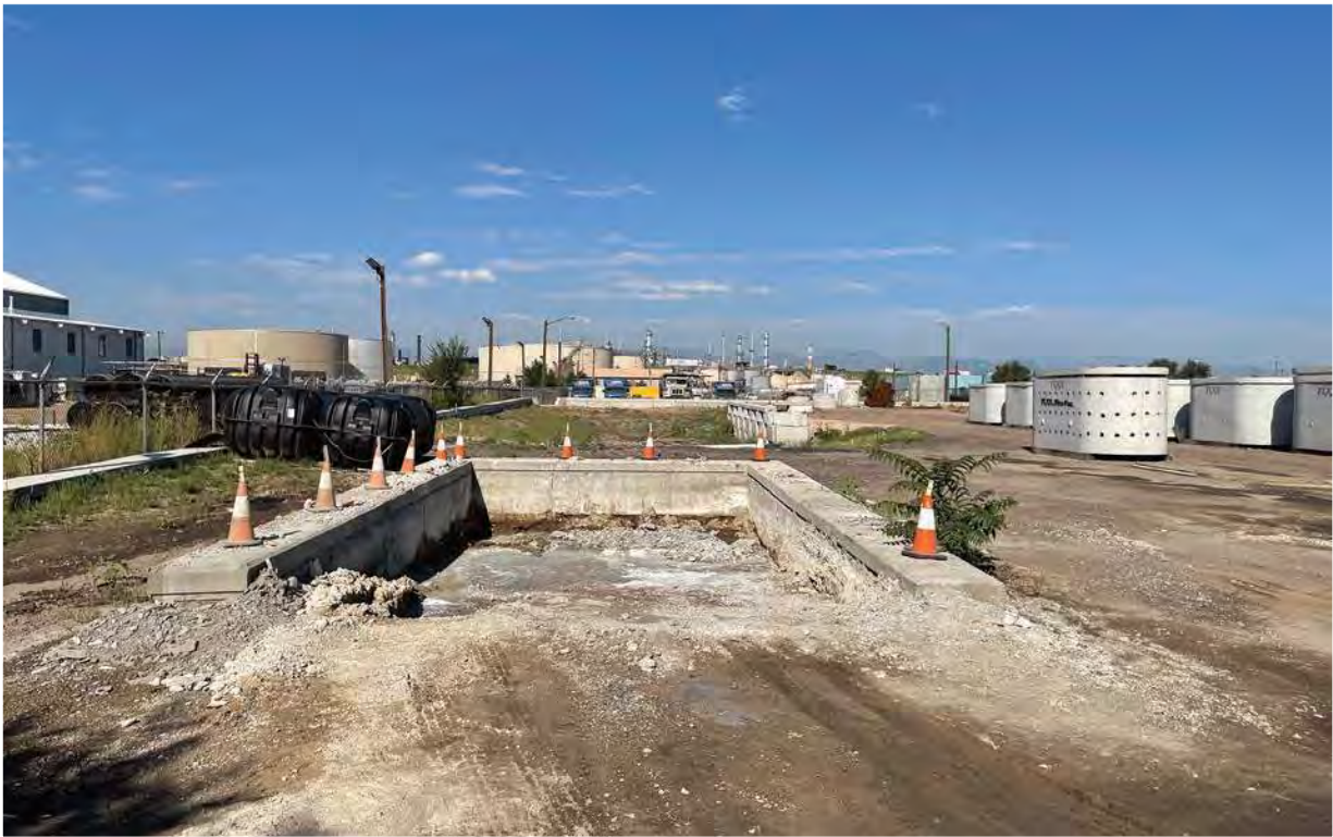
Photo 2 - A concrete washout observed in the Project Area at 5901 Dexter Street
